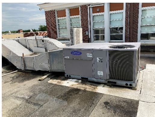
Applegarth School – Roof Top Unit
