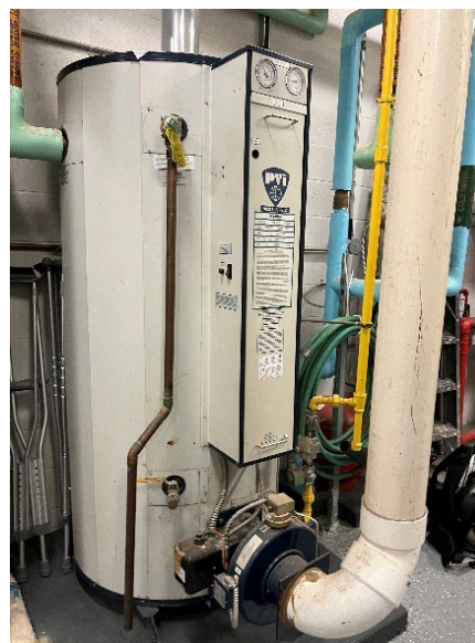
Woodland School – Water Heater
