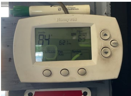
Garage Thermostat (AHU)
