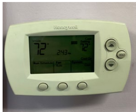
Programmable Thermostat (AHU)
