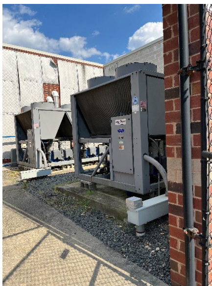
Oak Tree School - Chiller
