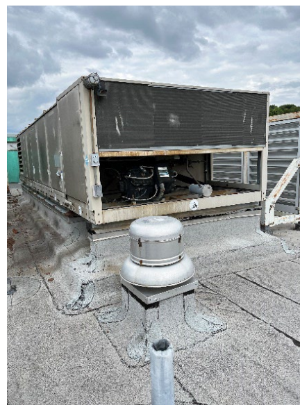
Mill Lake School Complex - RTU
