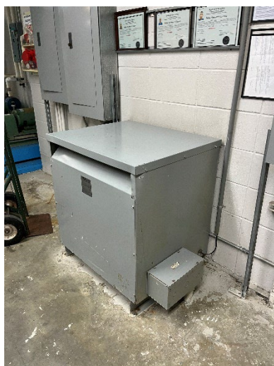
Barclay Brook School - Transformer
