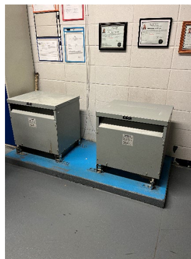
Mill Lake School Complex-Transformer
