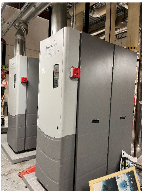
Oak Tree School - Boilers
