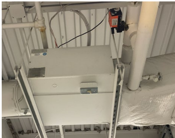
Typical VAV Box with DDC
