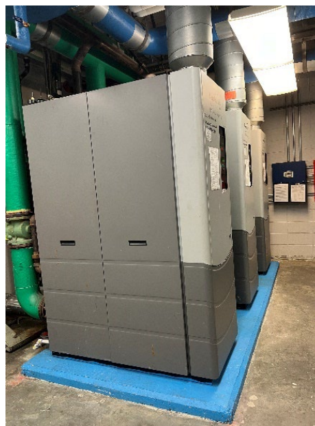
Barclay Brook School - Boilers
