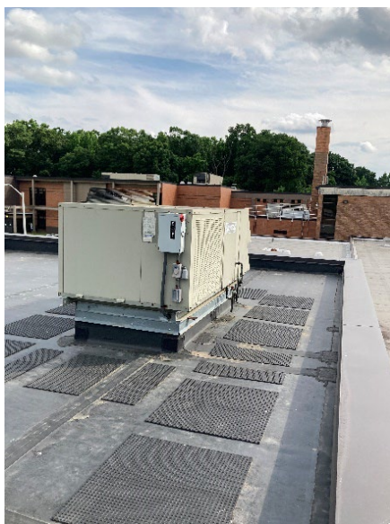
Monroe Twp. Middle School - RTU
