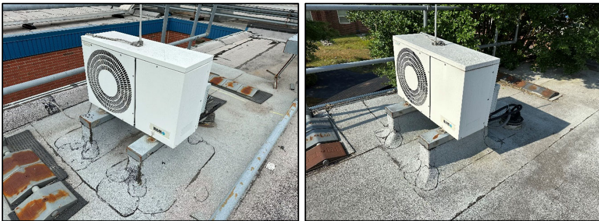
Existing split system AC units at Gloucester High School
