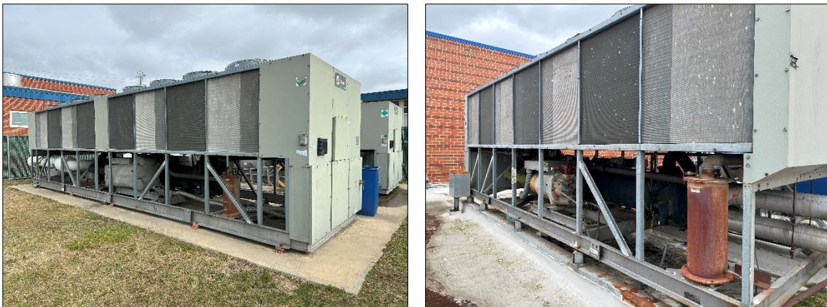
Existing air-cooled chiller at Gloucester HS and Cold Springs ES & ECC
