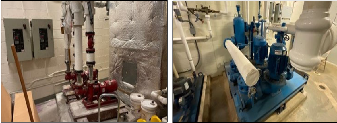
Pipe and valve insulation at Moore School and Woodruff School
