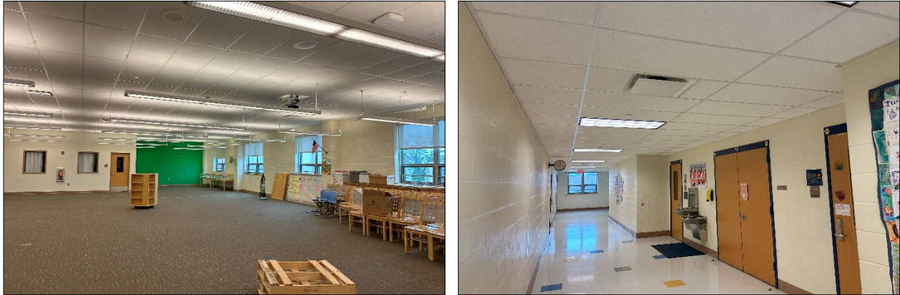
Existing interior lighting at Gloucester MS
