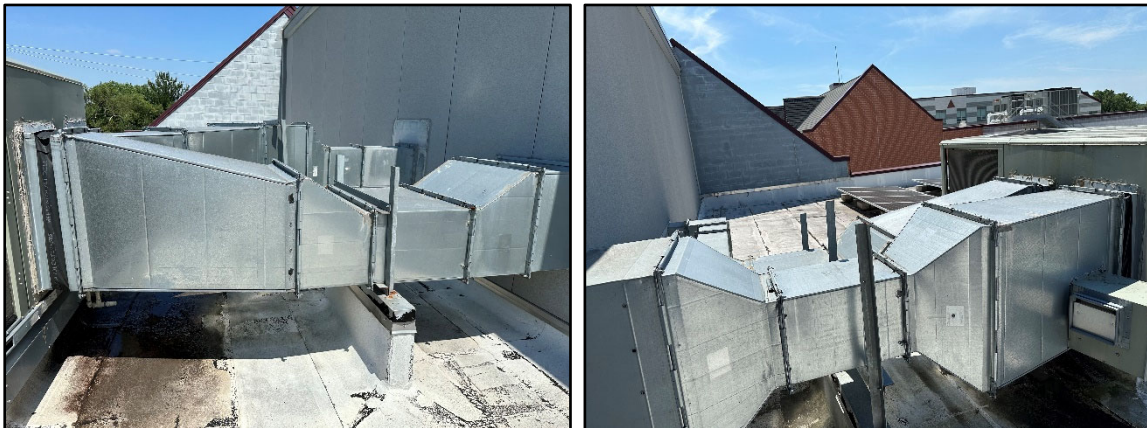
Existing exterior ductwork at Gloucester Middle School
