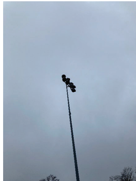
Haddonfield Memorial High School - Stadium Lighting
