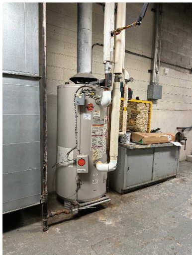
Haddonfield Middle School – Water Heater
