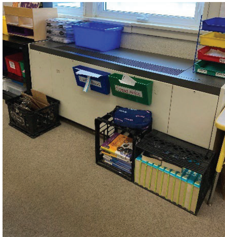
Elizabeth Haddon Elementary School – Unit Ventilator
