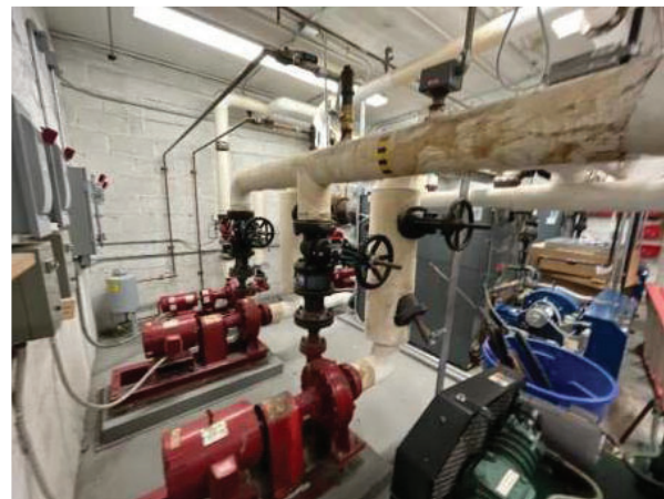
J. Fithian Tatem Elementary School - Pipe Insulation
