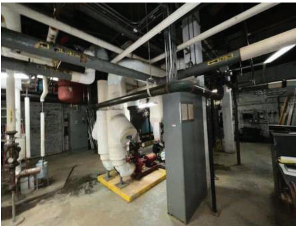
Haddonfield Memorial High School - Pipe Insulation
