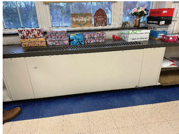
Haddonfield Middle School – Unit Ventilator
