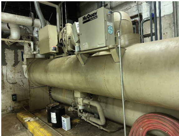
Haddonfield Memorial High School - Chiller
