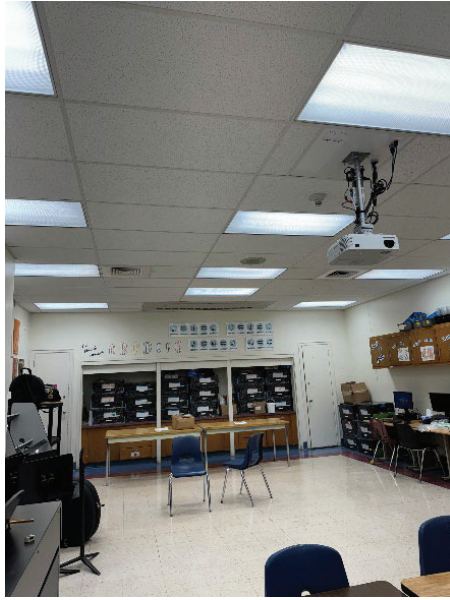
Lighting at Haddonfield Middle School
