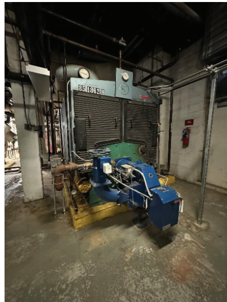
Haddonfield Memorial High School - Boilers
