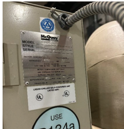
Haddonfield Memorial High School – Chiller
