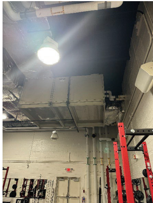
Haddonfield Memorial High School - AHU
