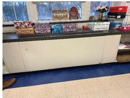
Haddonfield Middle School – Unit Ventilator
