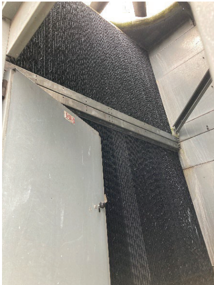
Haddonfield Memorial High School - Cooling Tower
