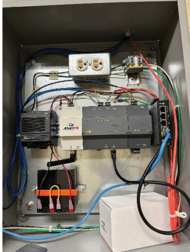
Haddonfield Memorial High School DDC Controls
