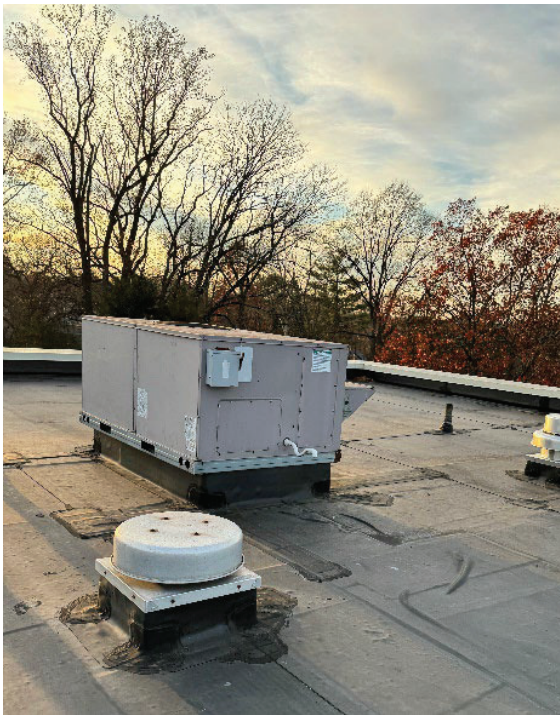
Haddonfield Memorial High School - RTU
