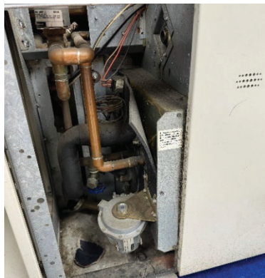
Haddonfield Middle School – Unit Ventilator
