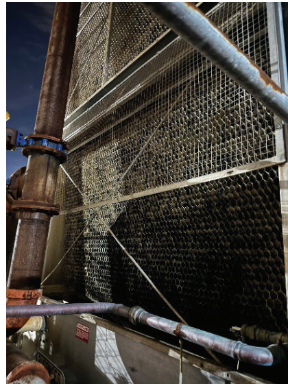
Haddonfield Memorial High School – Cooling Tower
