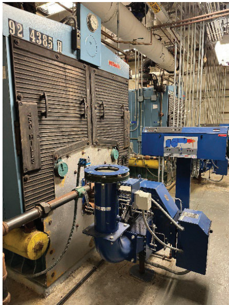
Haddonfield Middle School - Boilers
