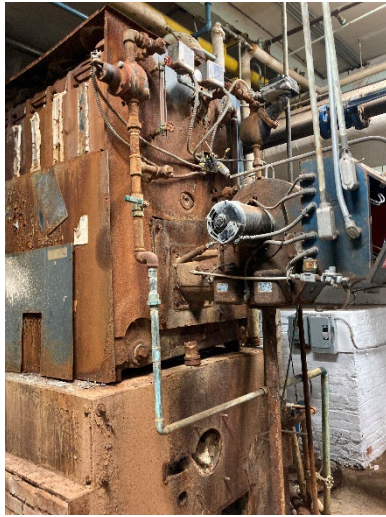
Oakwood Ave Community School - Boiler
