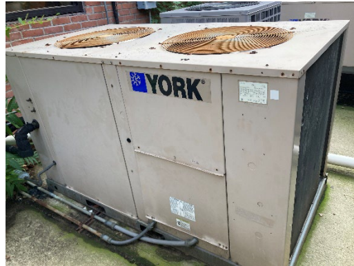
Administrative Offices – Split System
