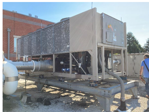
Park Avenue School – Chiller
