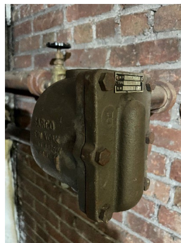
Central Elementary School - Steam Trap
