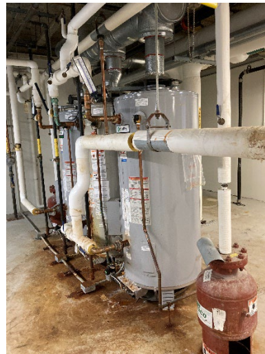
Rosa Parks Community School – Water Heater
