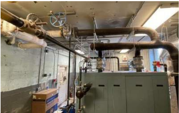
Forest Street ES - Pipe Insulation
