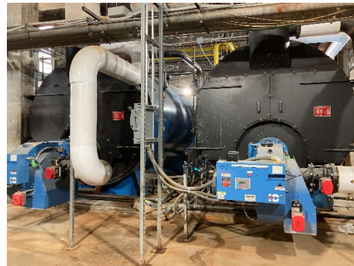
Orange High School and Prep Academy – Boiler Controls
