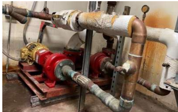
Oakwood ES - Pipe Insulation
