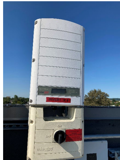
Park Avenue School - Solar Inverter
