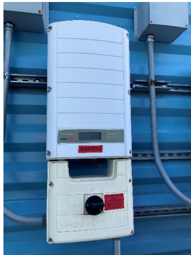
Lincoln Avenue School - Solar Inverter
