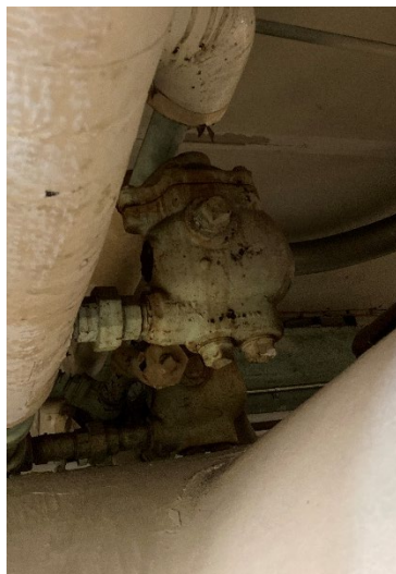
Oakwood Ave Community School – Steam Trap
