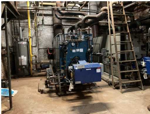
Central Elementary School - Boiler Controls
