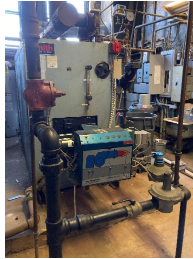
Scholars Academy - Boiler
