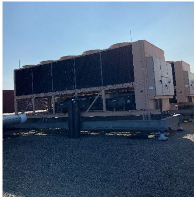
Rosa Parks Community School – Chiller
