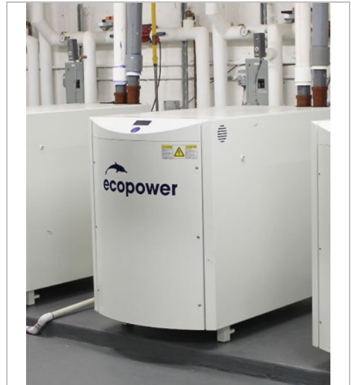
Axiom mCHP unit that consists of a reciprocating engine to generate electricity, and using the waste heat from the jacket.
