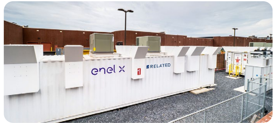
Figure 1-4. Related's Gateway Center battery storage system contributes to a cleaner, more efficient electric grid in its community.
