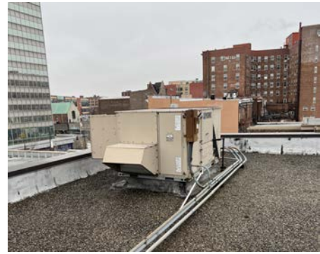
Figure 7. Existing RTU at CTC
