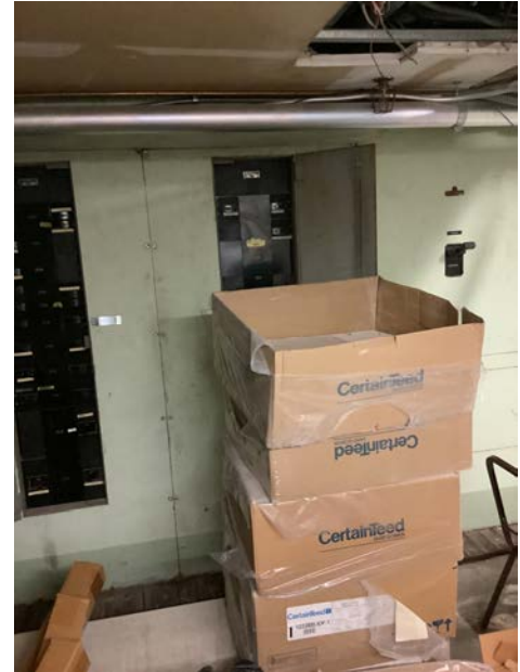
Figure 8. Existing Hamilton Hall Electrical Electrical switchgear requires replacement as systems degrade.
