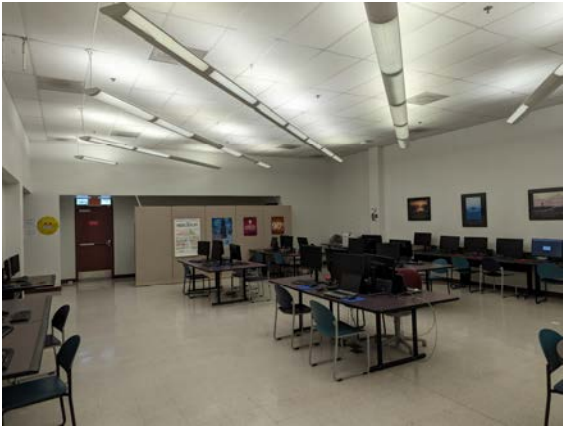
Figure 1. Existing Lighting at Wanaque Campus
