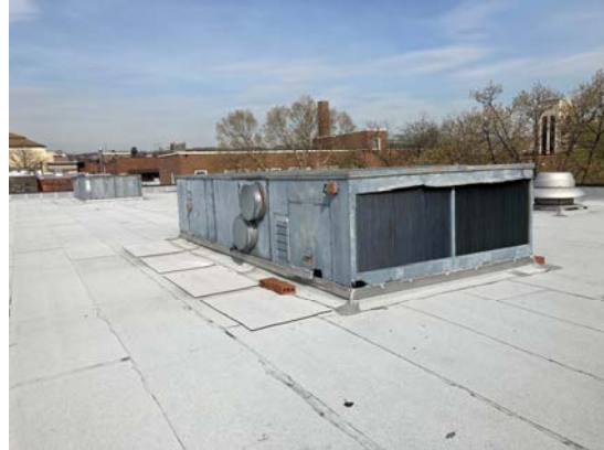
Figure 6. Existing heating only RTU
