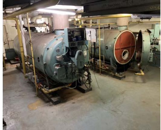
Figure 3. Existing HW boilers
