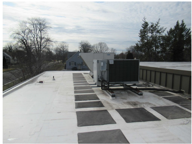
Existing packaged and split system units at Westergard Library
