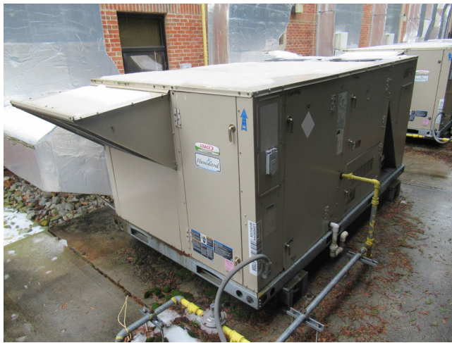
Existing packaged units (RTUs) at JFK Library.
