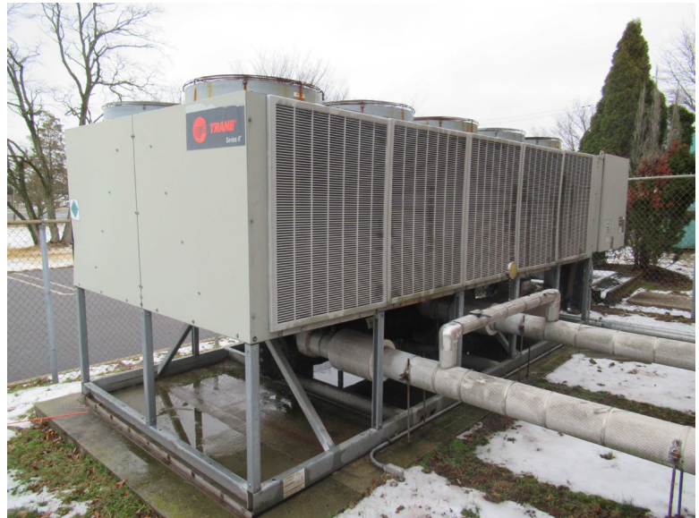
Existing air-cooled chiller at JFK Library.
