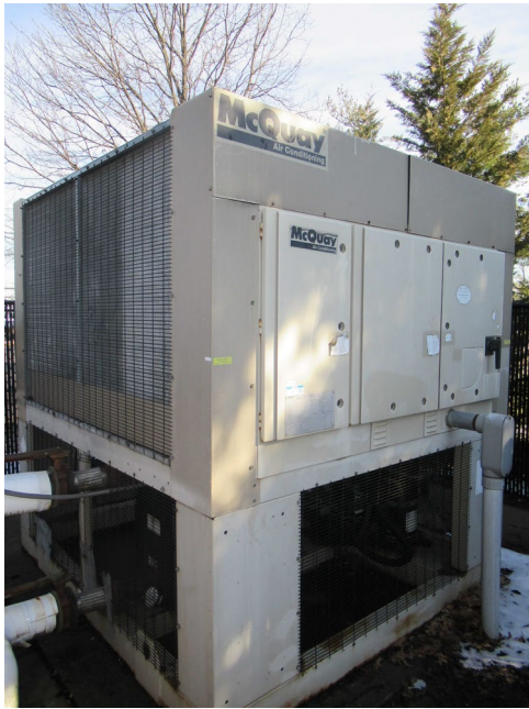
Existing air-cooled chiller at the Town Hall.
