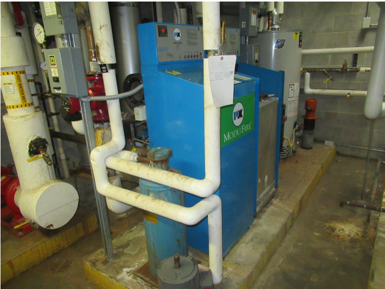
Existing non-condensing boilers at JFK Library.
