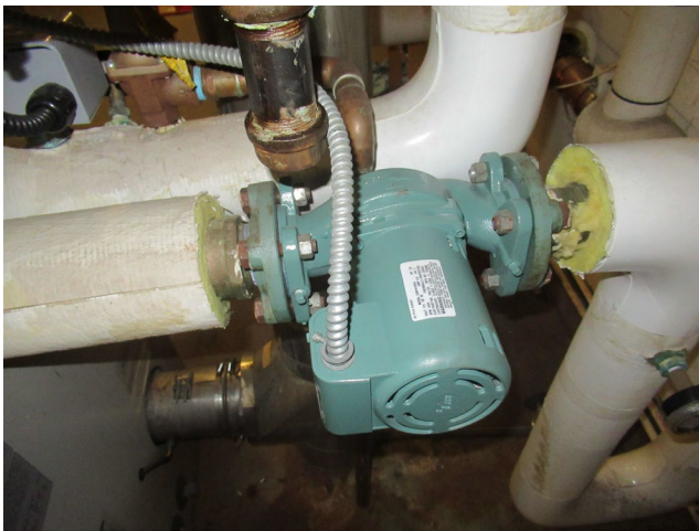
Existing boiler circulation pump at DPW (typical of 2).
