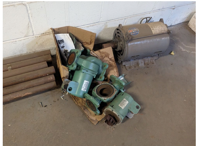
Pile of recently replaced boiler circulation pumps.
