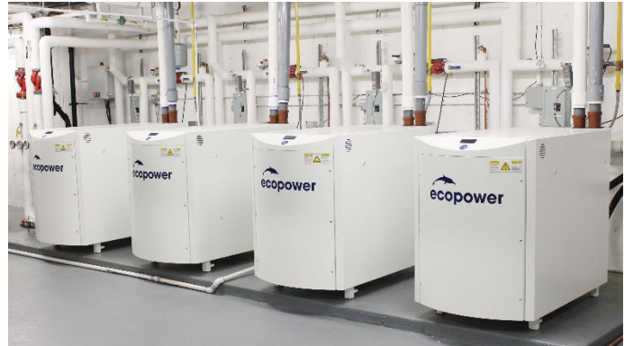
4.4kW Micro-combined CHP
