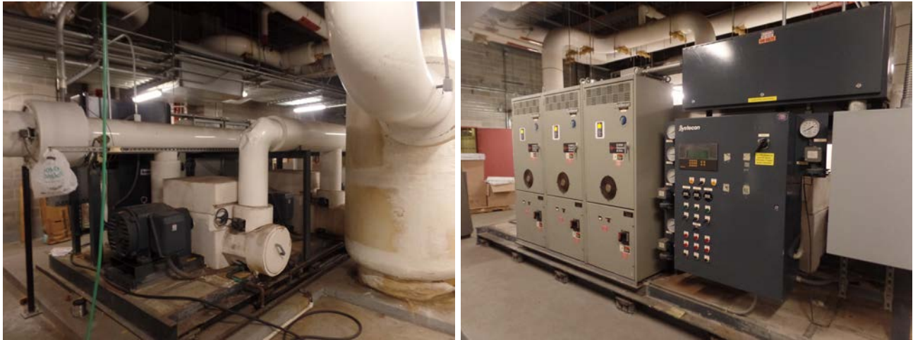
Existing booster pump skids located in the ACCC Mechanical Penthouse
