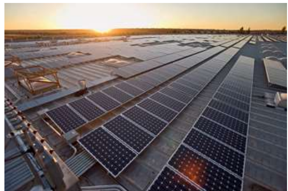
Photovoltaic (PV) solar array
