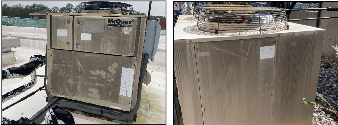
Existing split system condensers at Conover Road Elementary School
