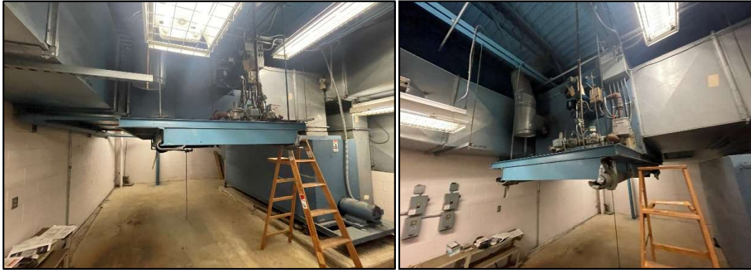
Existing AHU serving Conover Road ES Gymnasium
