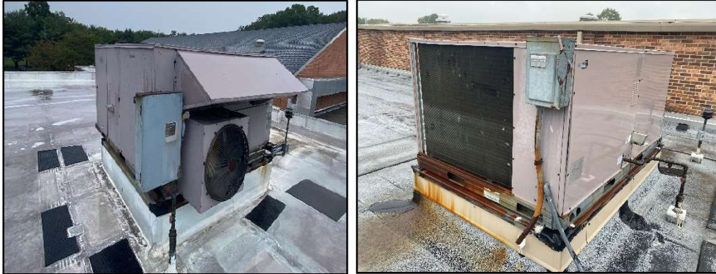
Existing RTUs at Cedar Drive MS and Conover Road ES
