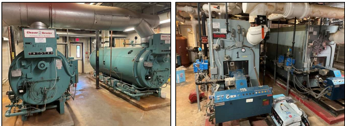
Existing boilers at Conover Road Primary School and Conover Road Elementary School
