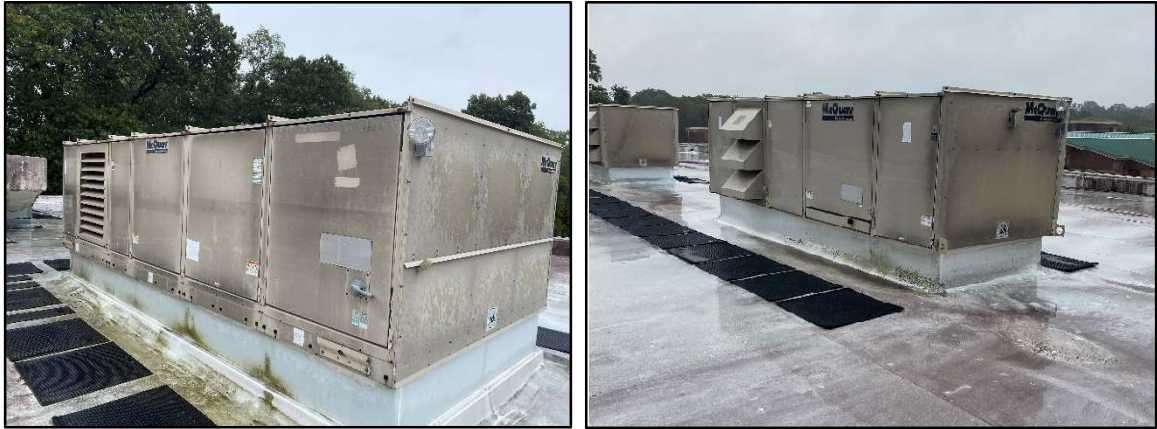
Existing H&V units at Cedar Drive MS and Conover Road ES
