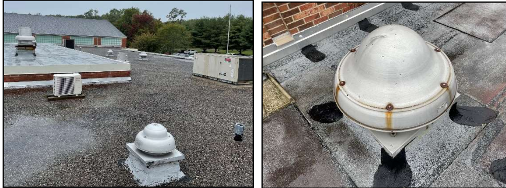
Existing exhaust fans at Cedar Drive MS and Conover Road ES
