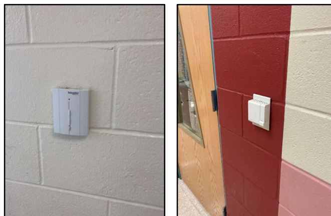
Existing controls at Conover Road ES & Conover Road PS
