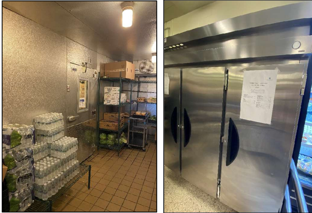
Existing freezer/ refrigeration equipment at Conover Road PS & Cedar Drive MS
