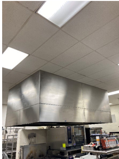
Clearview Regional HS - Kitchen Hood
