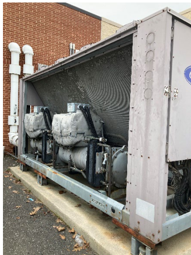
Clearview Regional HS - Chiller
