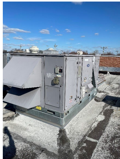
Clearview Regional HS - RTU
