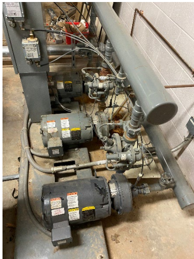
Clearview Regional HS – Domestic Water Pump Skid
