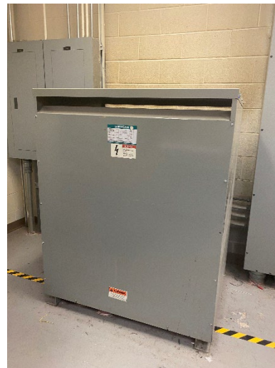
Clearview Regional HS - Transformer
