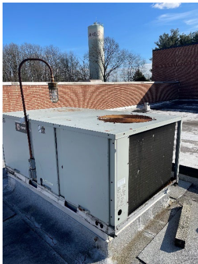
Clearview Regional HS - RTU
