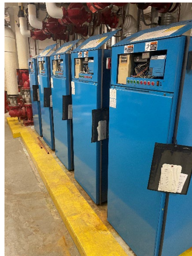
Clearview MS - Boiler
