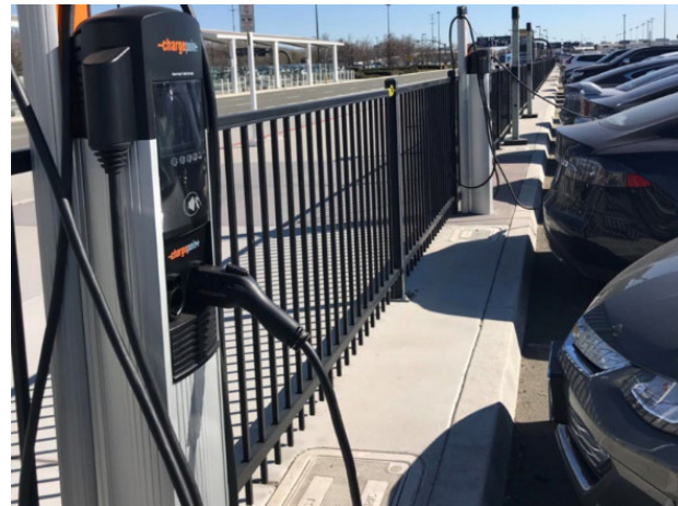
Sample Level 2 EV Chargers
