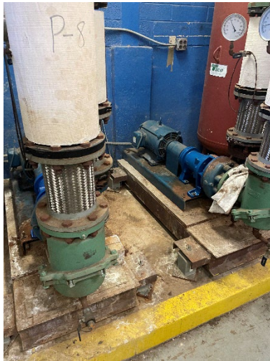
Clearview Regional HS – Motor
