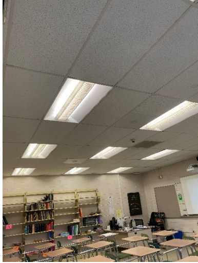
Lighting at Clearview Regional HS
