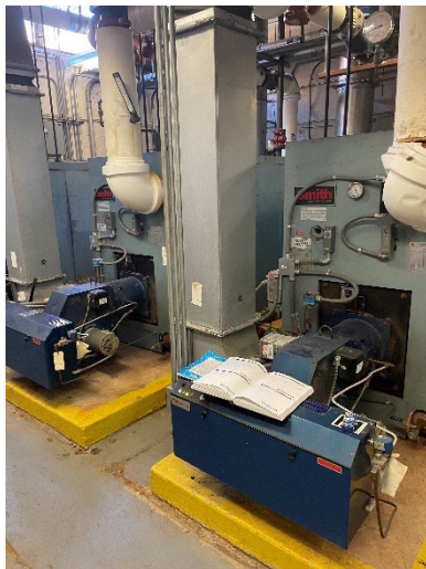
Clearview Regional HS - Boiler
