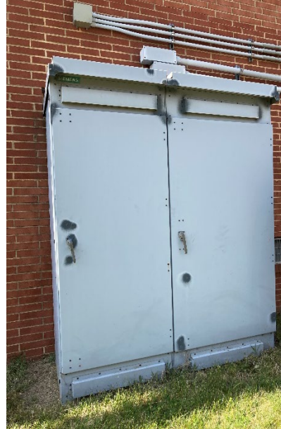
Switchgear at Clearview MS
