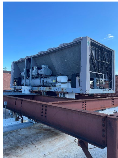
Clearview Regional HS - Chiller
