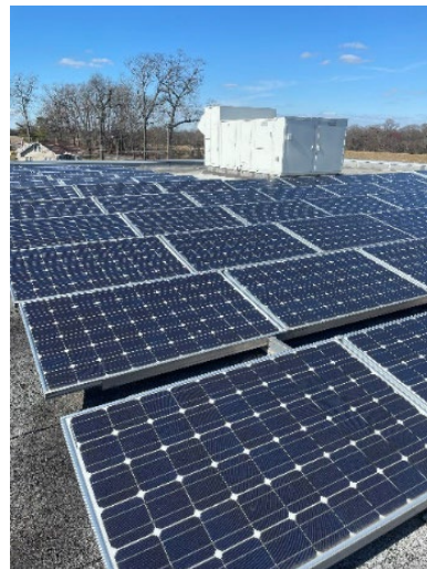
Clearview MS - Existing Solar Arrays
