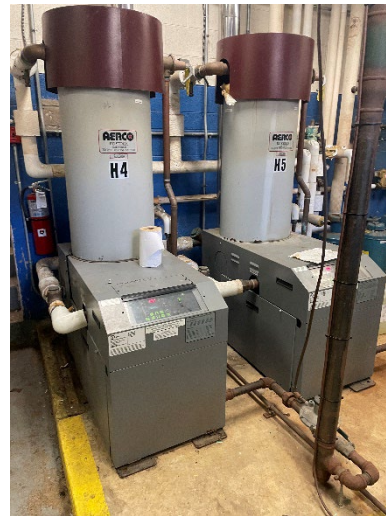
Clearview Regional HS – Water Heater
