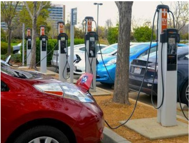
Sample Level 2 EV Chargers
