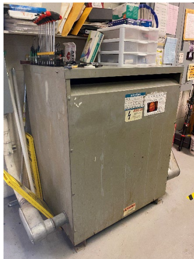
Clearview Regional HS - Transformer
