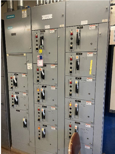
Switchgear at Clearview Regional HS
