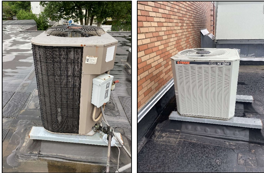
Existing split system AC units at Honiss School and Grant School
