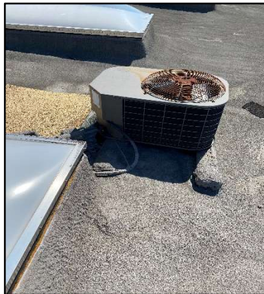
Existing Split system AC unit at Dumont HS
