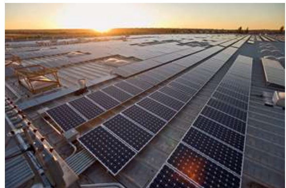
Photovoltaic (PV) solar array
