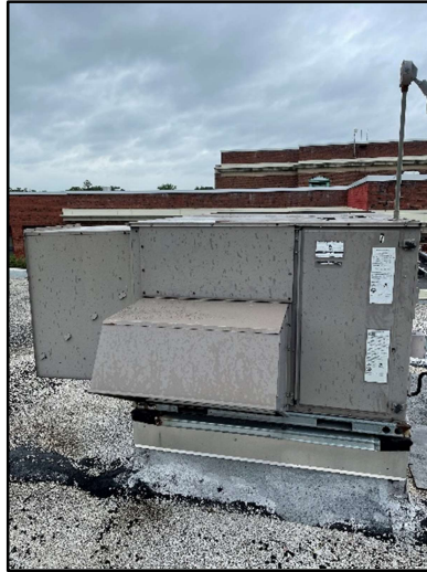
Existing roof top units at Dumont HS
