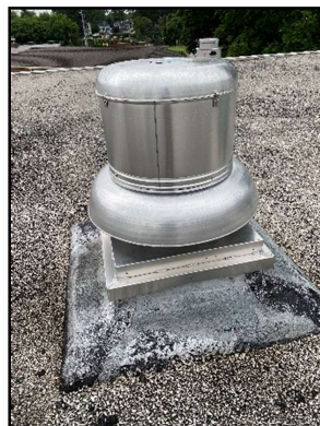
Existing exhaust fans at Dumont HS
