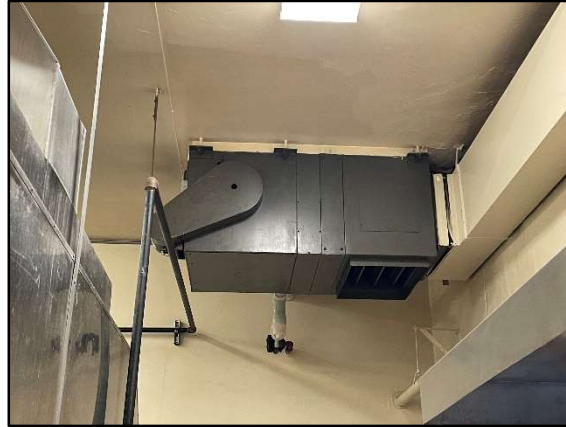
Existing AHU at Dumont HS
