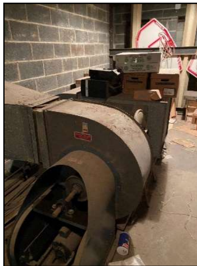
Existing AHU at Honiss School
