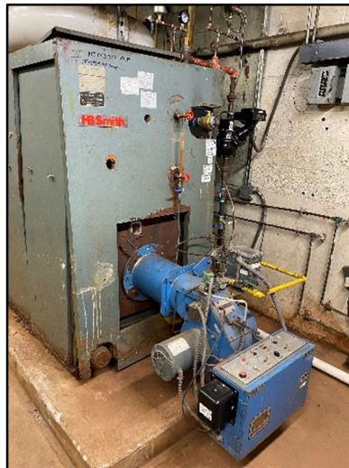
Existing force draft steam boilers at Honiss School
