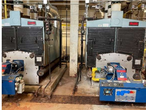
Existing force draft steam boilers at Dumont HS
