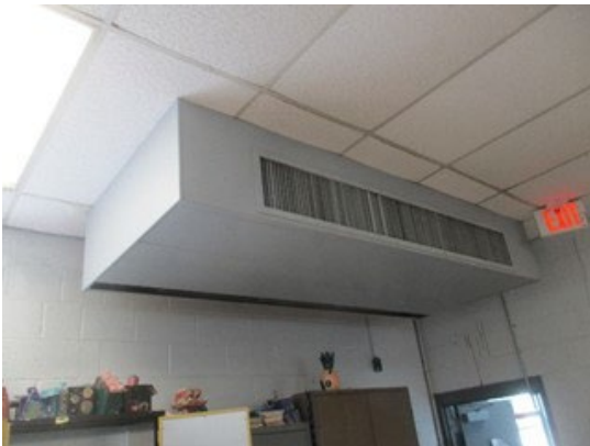
Industrial Arts Building – Unit Ventilator
