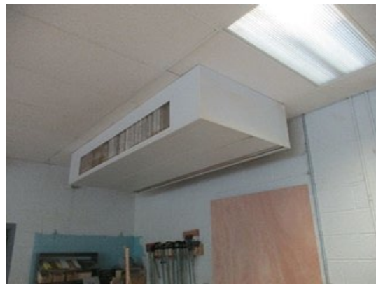
Industrial Arts Building – Unit Ventilator
