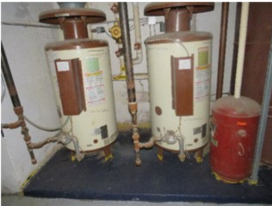
Manasquan High School – Water Heaters
