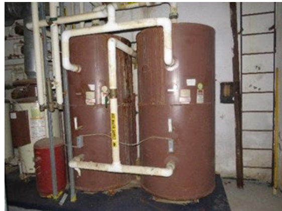
Manasquan High School – Storage Tanks
