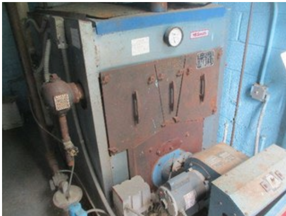
Industrial Arts Building - Boiler
