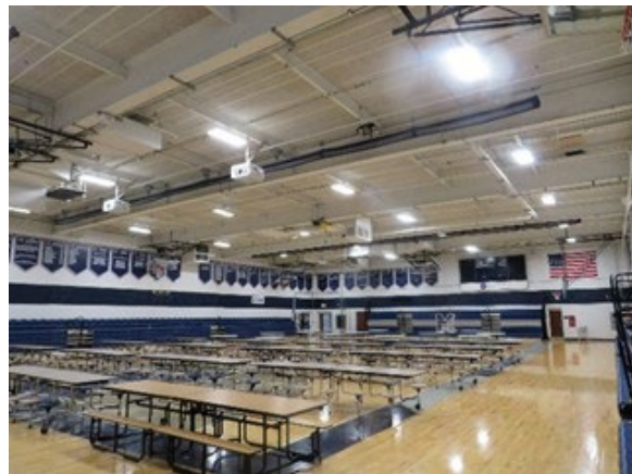
Lighting Control Space at Manasquan HS
