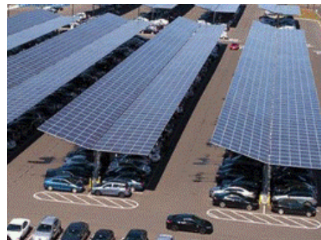
Typical Parking Lot Solar Array
