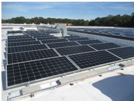
Typical Rooftop Solar Array
