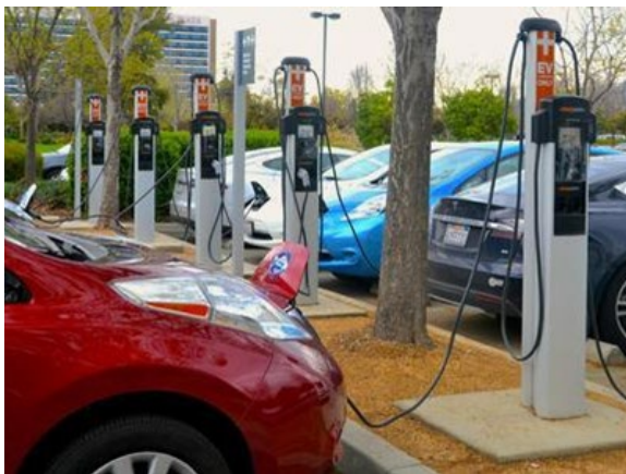
Sample Level 2 EV Chargers
