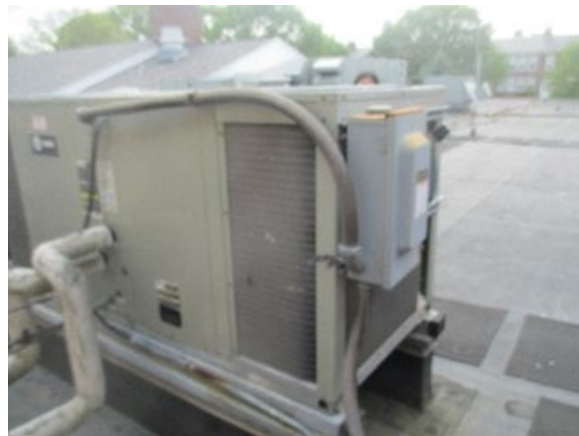
Manasquan Elementary School – Split System
