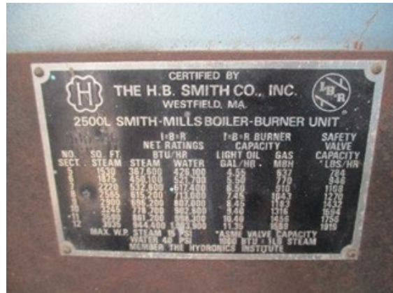
Industrial Arts Building - Boiler
