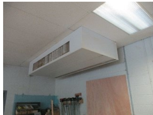
Industrial Arts Building – Unit Ventilator
