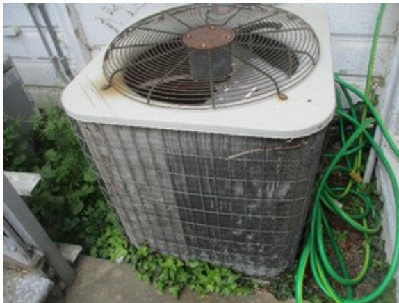
Administrative Building – Split System
