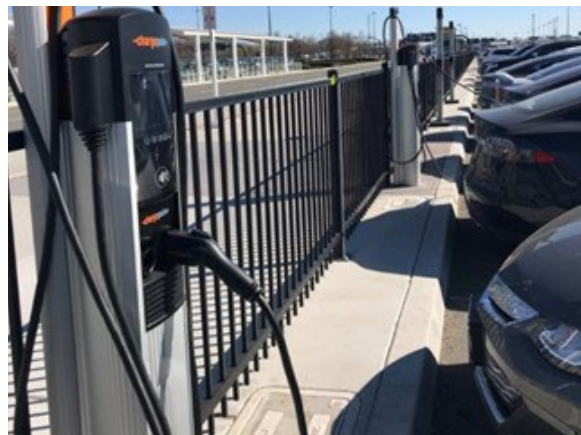
Sample Level 2 EV Chargers
