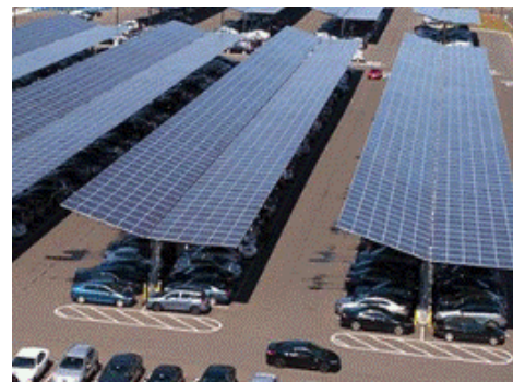
Typical Parking Lot Solar Array
