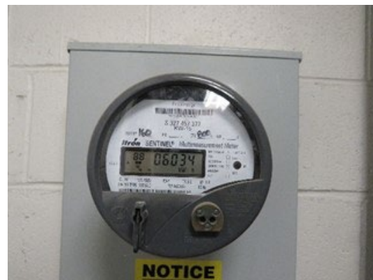
Manasquan HS - Electric Meter
