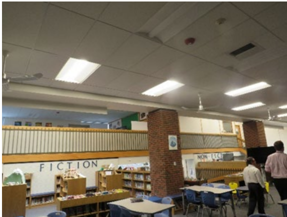
Existing Lighting at Manasquan ES
