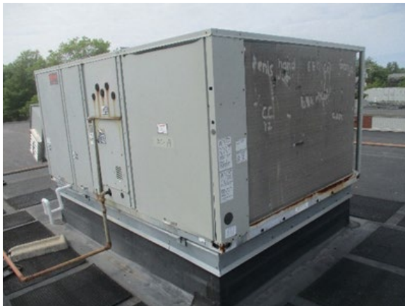
Manasquan Elementary School RTU
