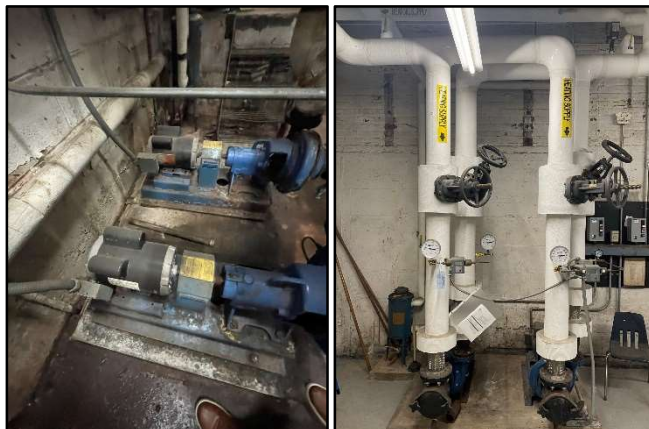
Existing Pumps and Motors at Slocum Skews and Bergen Blvd
