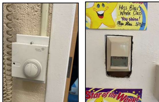
Existing pneumatic controls at Memorial High School and Bergen Blvd
