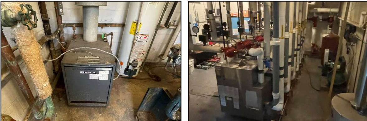
Existing hot water boilers at Central Office and Shaler Academy
