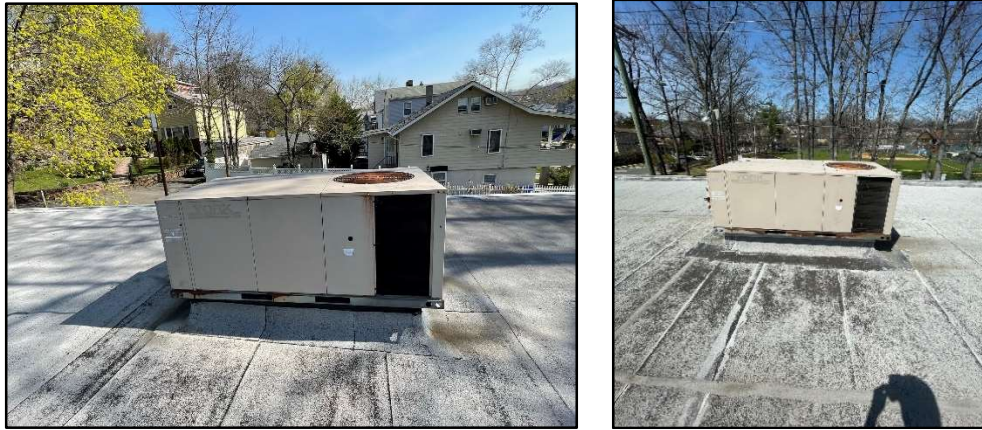
Existing Heat Pumps at Shaler Academy and Memorial High School
