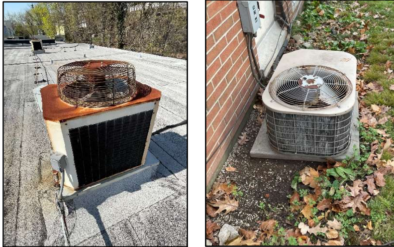
Existing AC Units at Shaler Academy and Central Office
