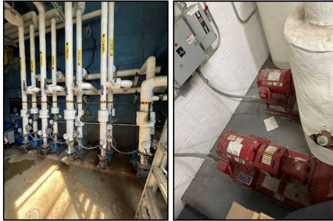
Existing Pumps and Motors at Memorial High School and Shaler Academy
