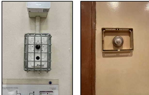
Existing pneumatic controls at Slocum Skews School and Shaler Academy
