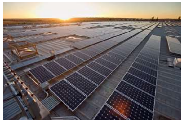
Photovoltaic (PV) solar array
