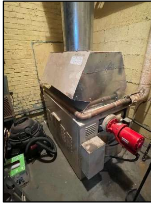
Existing Water Heater at Memorial High School
