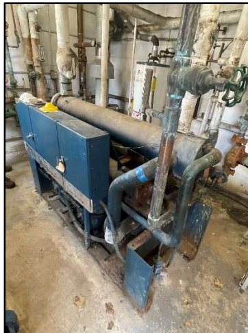
Existing chiller at Central Office
