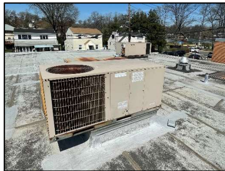
Existing Rooftop Units at Memorial High School
