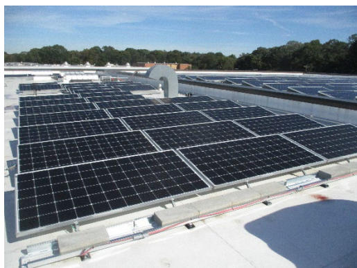
Typical Rooftop Solar Array
