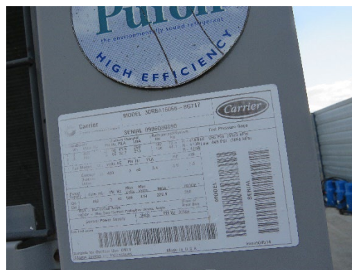
Chiller – Burlington City HS
