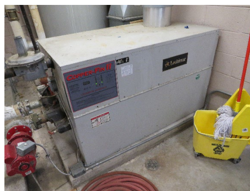
Wilber Watts IS – Water Heater
