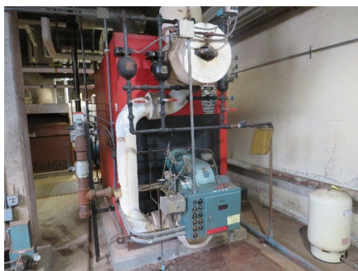
Captain James Lawrence ES - Boiler
