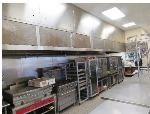
Burlington City HS - Kitchen Hood
