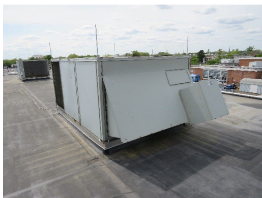
Burlington City HS - RTU
