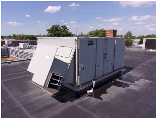
Burlington HS RTU
