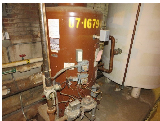
Samuel Smith ES – Water Heater
