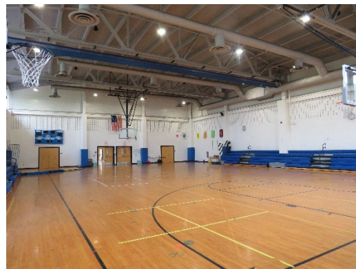
Lighting Control Space At Wilber Watts IS
