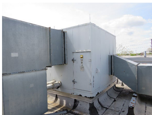
AHU – Burlington City HS
