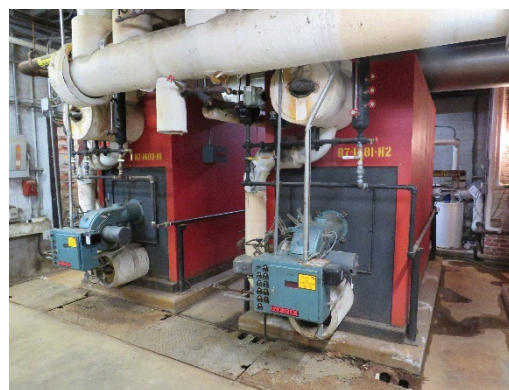
Samuel Smith ES - Boiler
