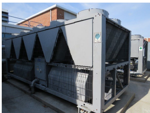
Chiller – Burlington City HS
