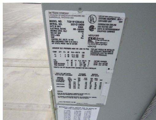
Burlington City HS - RTU
