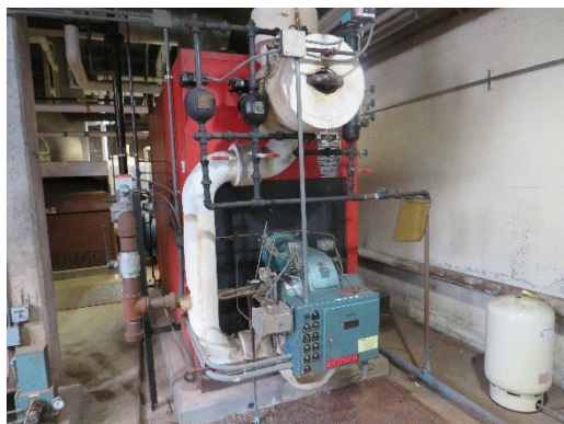
Captain James Lawrence ES - Boiler
