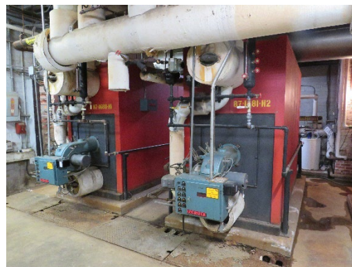
Samuel Smith ES - Boiler
