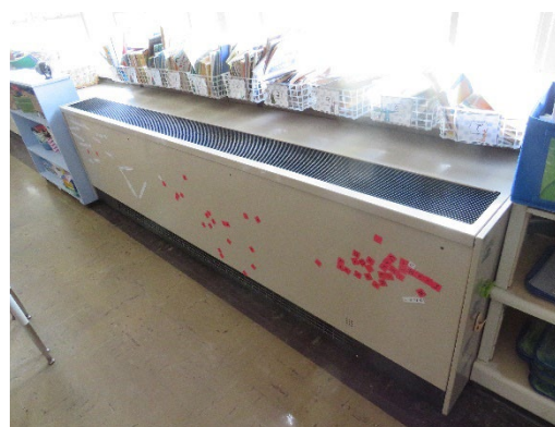
Captain James Lawrence ES – Unit Ventilator
