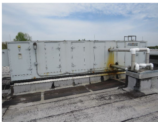
Wilber Watts IS - AHU
