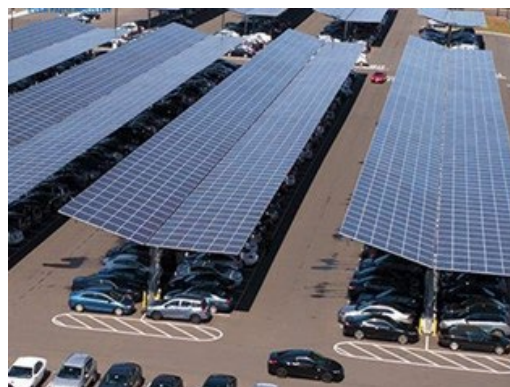
Typical Parking Lot Solar Array
