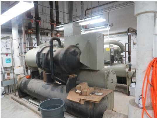
Chiller – Fernwood Ave MS
