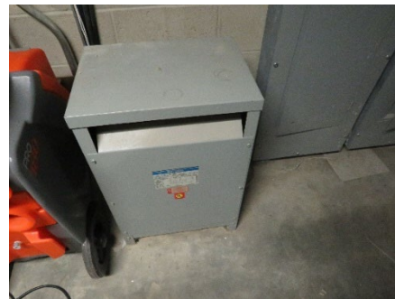
Alder Avenue MS - Transformer
