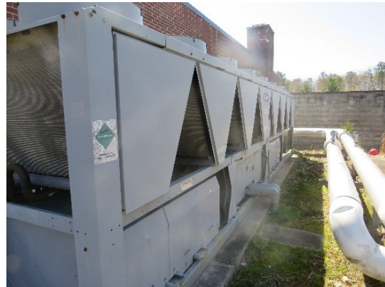
Chiller - Alder Avenue Middle School
