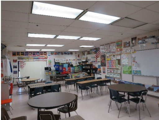
Existing Lighting at Fernwood Ave MS
