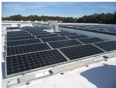
Typical Rooftop Solar Array
