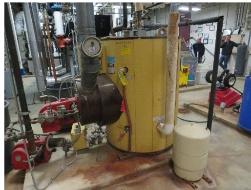
Alder Avenue MS – Water Heater
