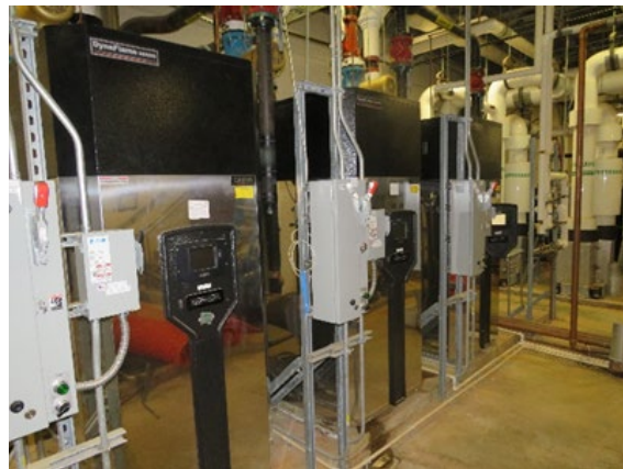
Alder Avenue MS - Boiler
