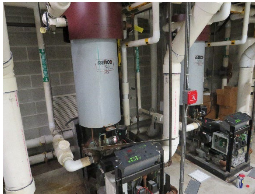
Egg Harbor Township HS – Water Heater
