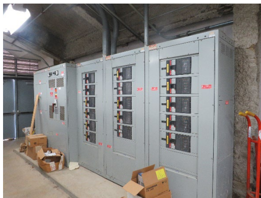
Fernwood Ave MS – Switchboard
