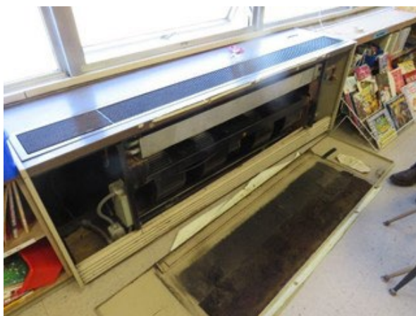
Martha B. Day School – Unit Ventilator
