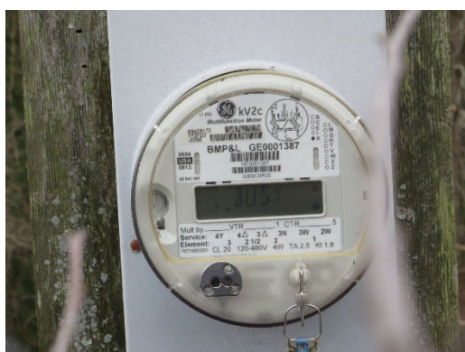
Samuel R. Donald School - Electric Meter
