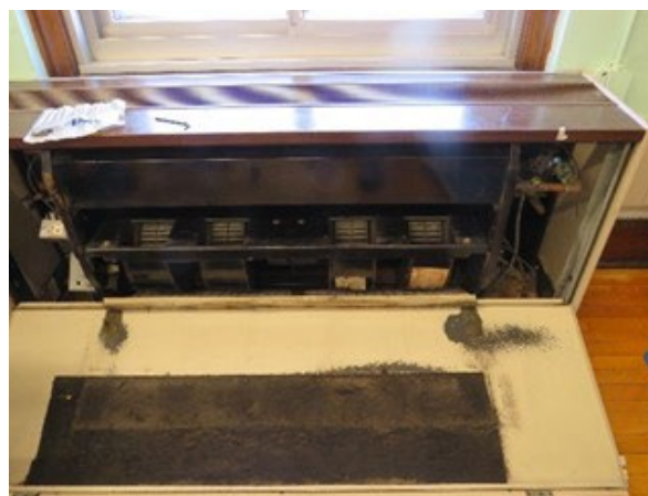
Samuel R. Donald School – Unit Ventilator
