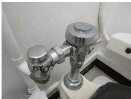
Samuel R. Donald School water fixtures
