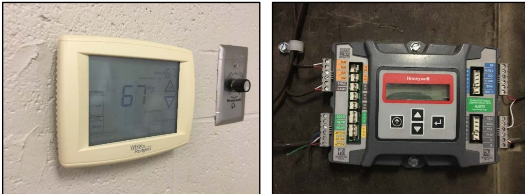
Existing thermostat at Roosevelt Elementary School and AHU controller at Lodi High School
