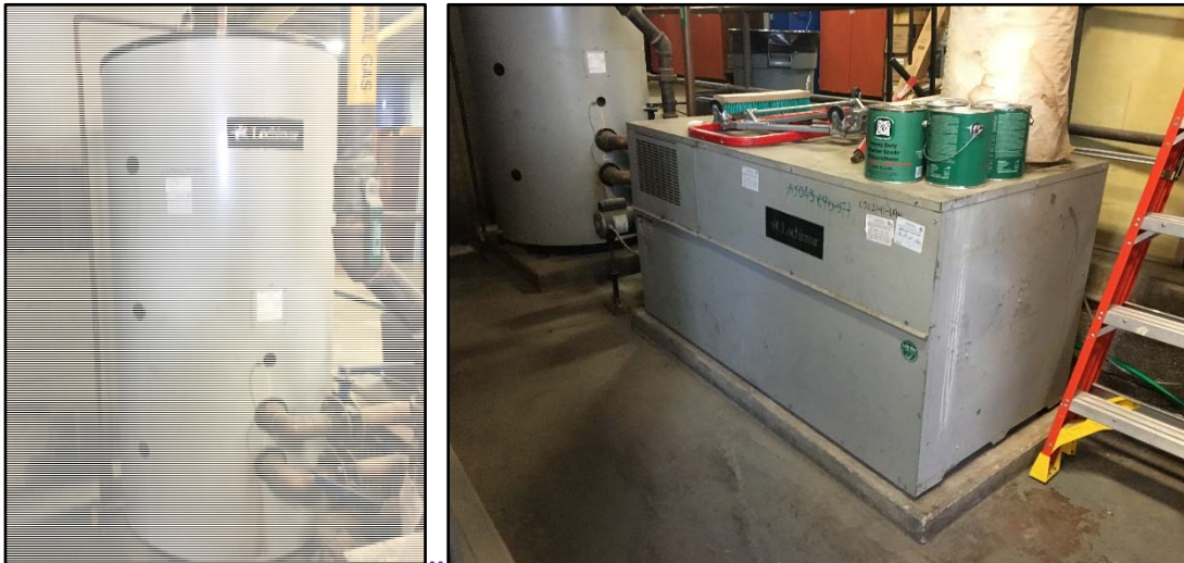
Existing Domestic Water Heater (Boiler and Tank) at Lodi High School
