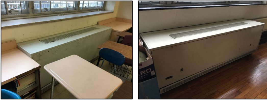
Existing unit ventilators at Thomas Jefferson Middle School and Washington Elementary
