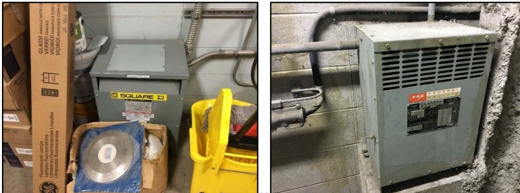
Existing Transformers at Lodi High School
