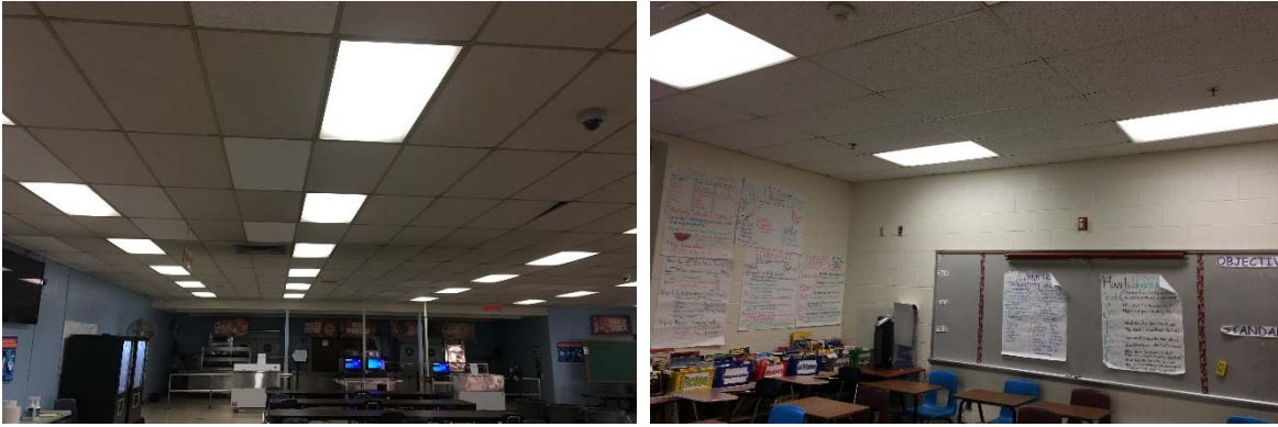
Existing interior lighting at Lodi HS and Thomas Jefferson MS
