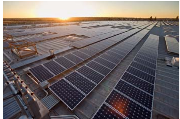
Photovoltaic (PV) solar array
