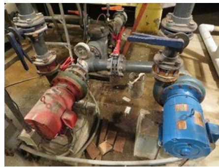
Washington MS Existing Pool Filter Pumps
