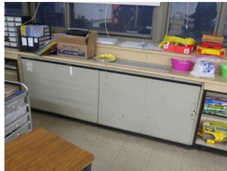
Lincoln ES – Typical Unit Ventilator
