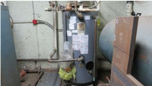
Hamilton Intermediate School Water Heater
