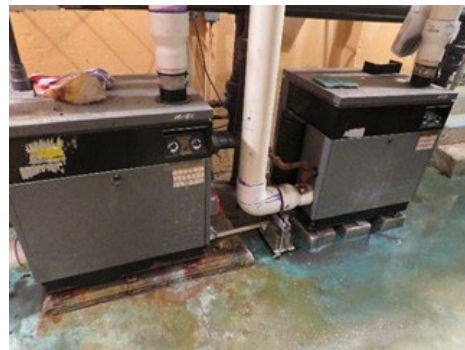
Washington Middle School Pool Water Heater
