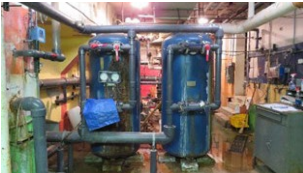
Washington MS Existing Pool Filters
