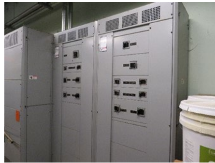
Harrison HS - Typical Electric Panel
