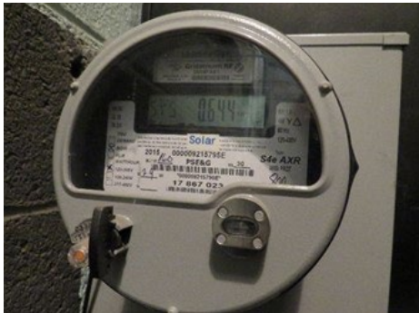
Washington MS - Typical Electric Meter
