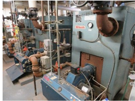
Lincoln Elementary School - Boilers
