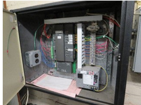
Lincoln School BMS Controller
