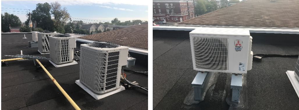
Existing split system AC units at the Administration Building
