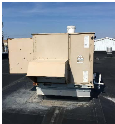
Existing gas fired RTU at the Administration Building
