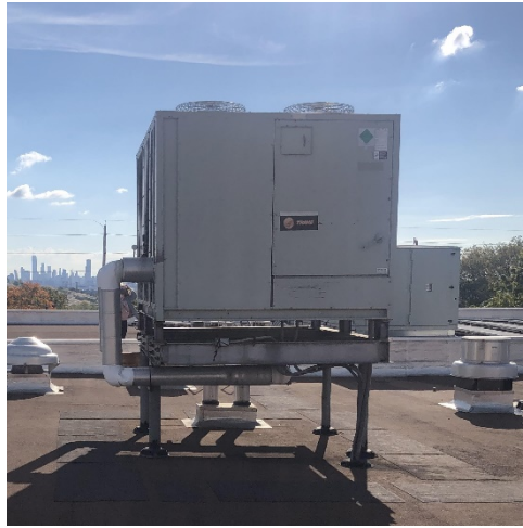
Existing chiller at Schuyler Elementary School
