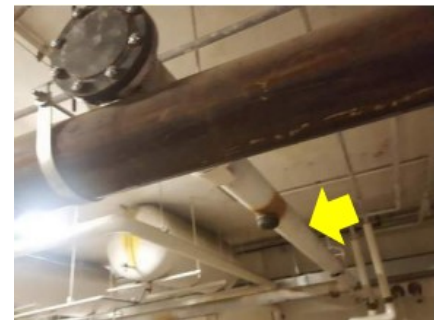
Uninsulated hot water piping
