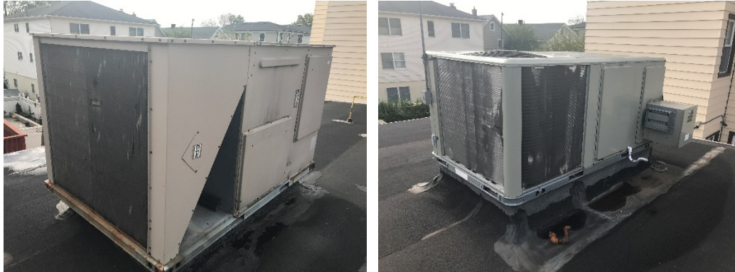
Existing roof top units at the Administration Building
