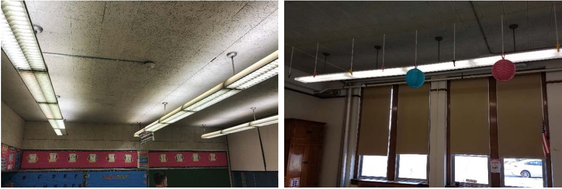
Existing interior lighting at Franklin and Garfield Elementary Schools
