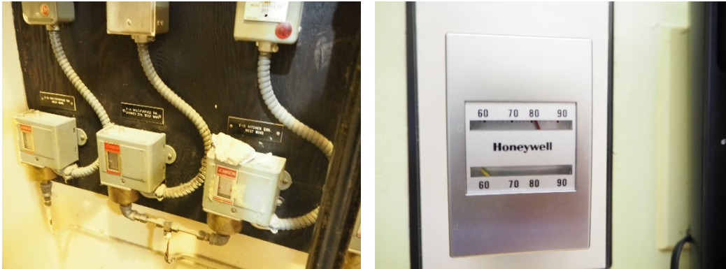
Existing pneumatic controls at Franklin Elementary School
