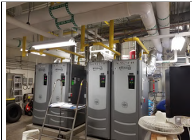
Hot Water Boilers
