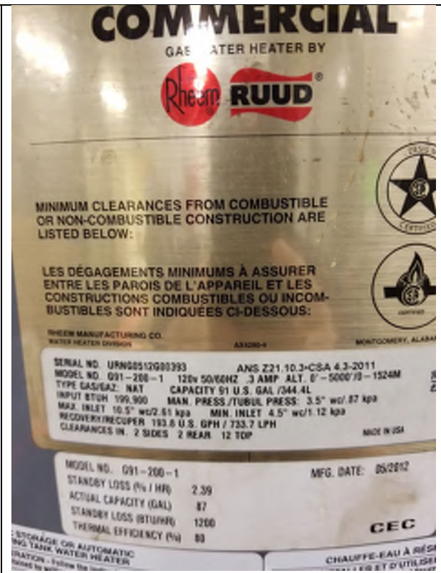
Domestic Hot Water Heater Nameplate
