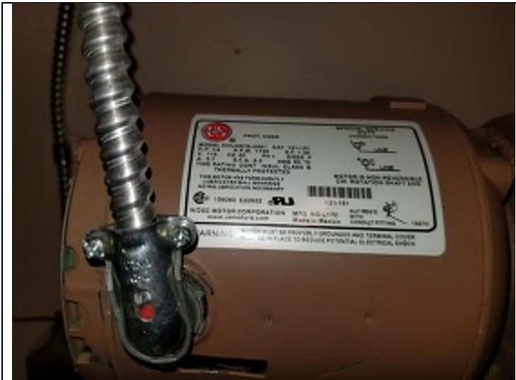
DHW Circulation Pump
