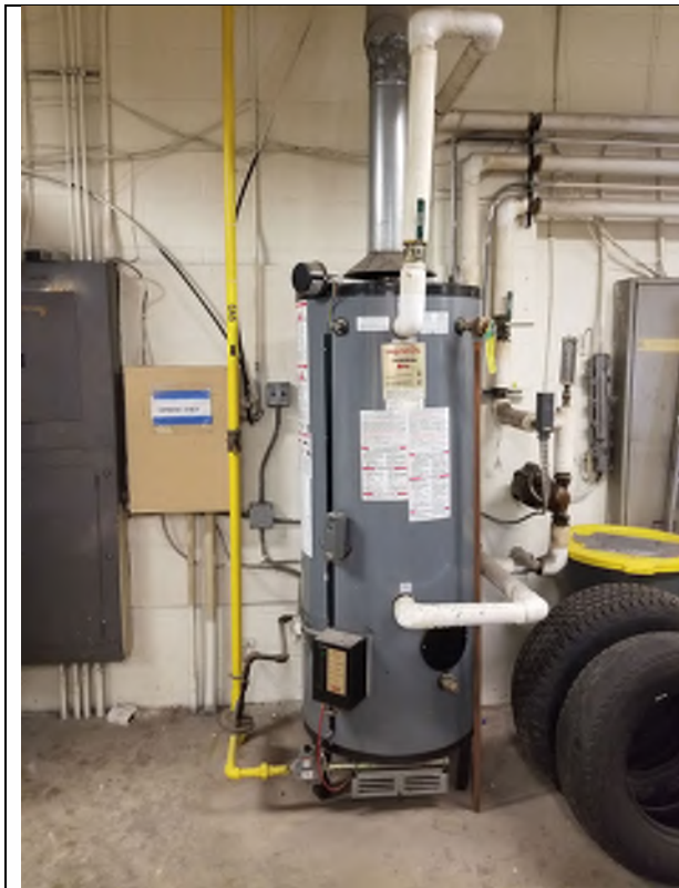
Domestic Hot Water Heater
