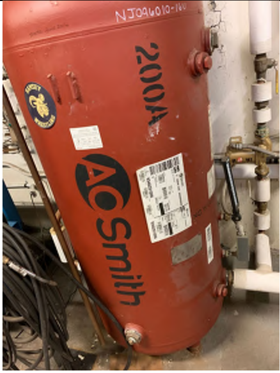
Domestic Hot Water Storage Tank Ramsey High School
