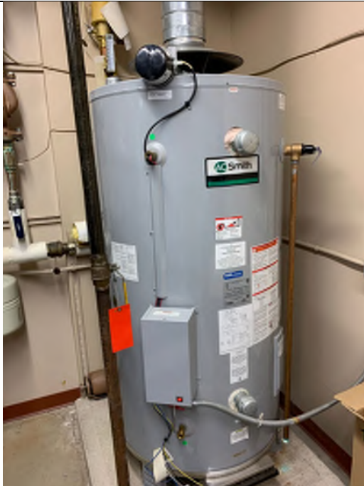
Domestic Hot Water Heater
