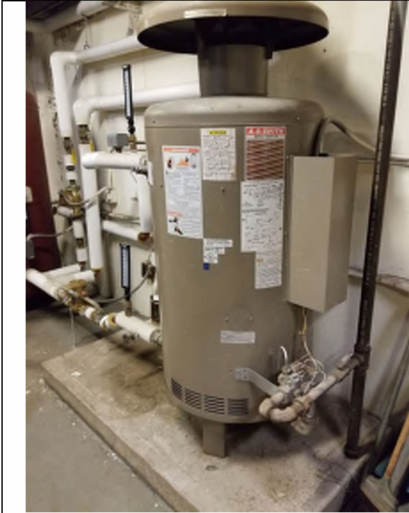
Domestic Hot Water Heater Ramsey High School
