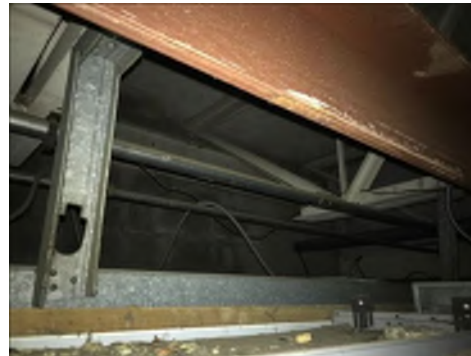
Overhang Air Sealing – there is no barrier separating the exterior overhang (area beyond metal framing) from the conditioned interior space
