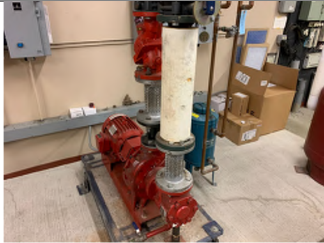
Heating Hot Water Pump
