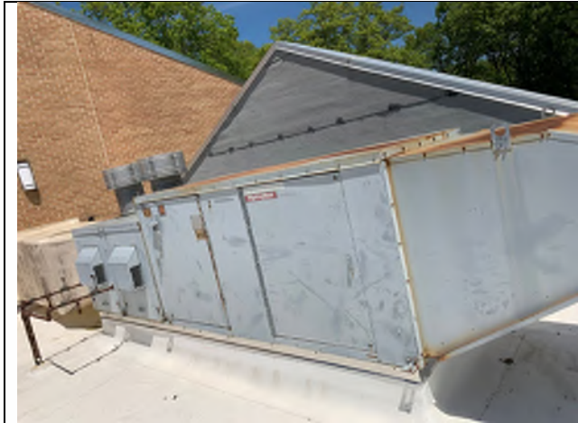
Make Up Air Units for Gymnasium
