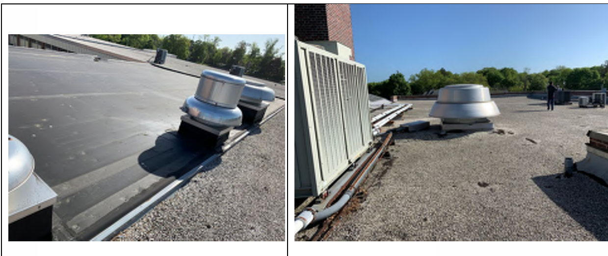
Existing Exhaust Fans
