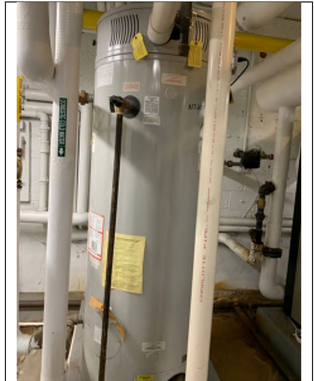
Domestic Hot Water Heater
