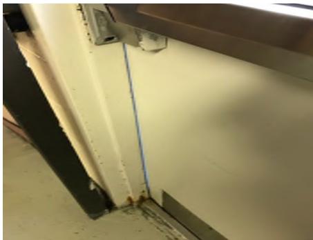
Door Weather Stripping – daylight showing through the sides of the door is a clear indicator that there is not a tight weather-stripping seal
