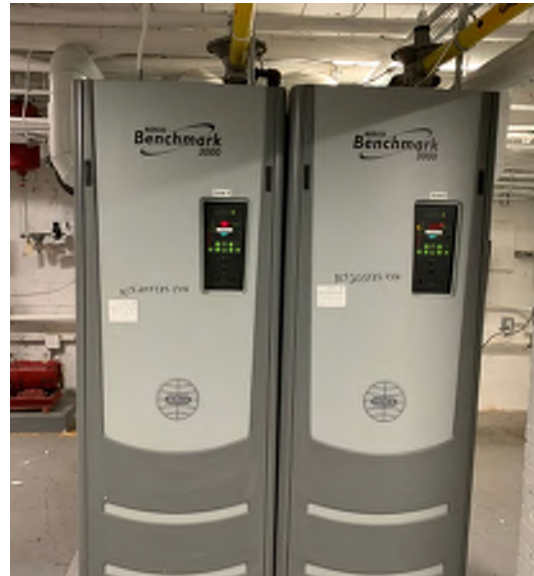
Hot Water Boiler
