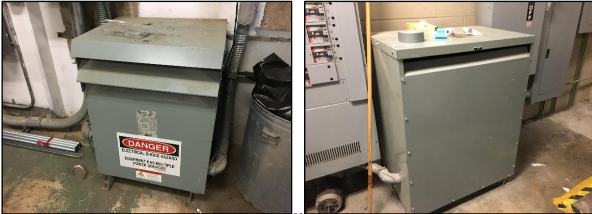
Existing Transformers at Ramapo HS and Indian Hills HS
