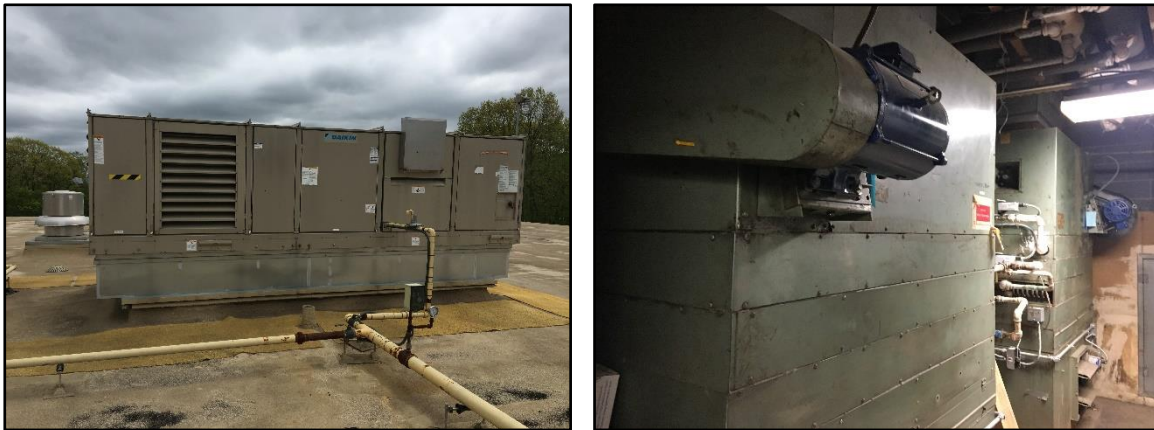
Existing unit rooftop H&V unit and internal AHU at Indian Hills HS
