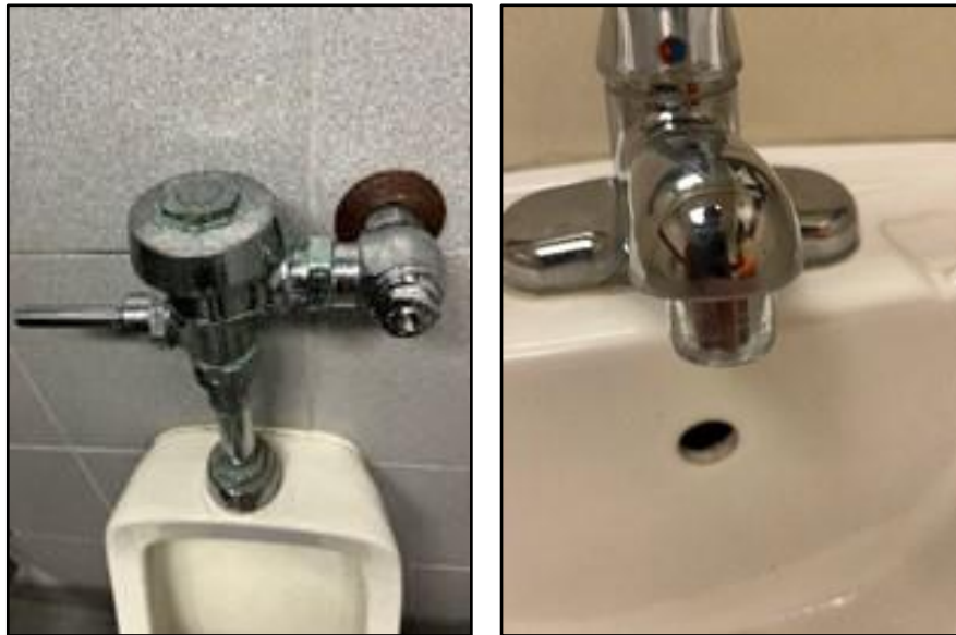
Existing equipment at Ramapo HS and Indian Hills HS
