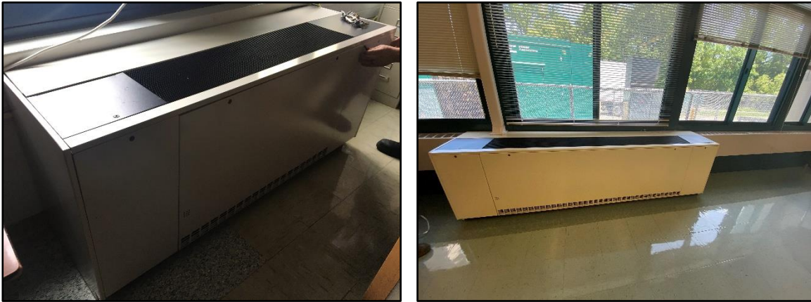
Existing unit ventilators at Indian Hills HS and Ramapo HS
