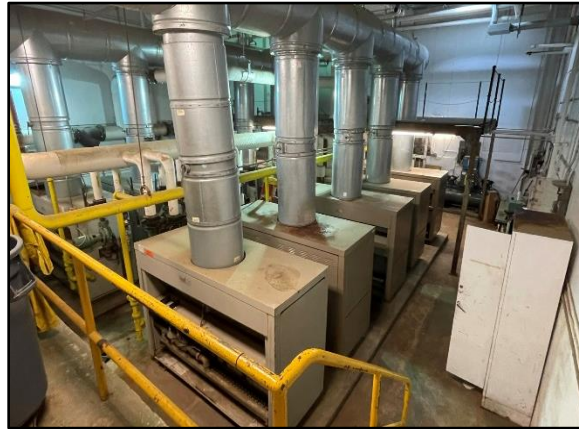
Hot water boilers before replacement at Ramapo High School
