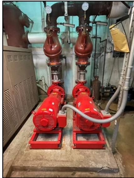
Hot Water Pumps before replacement at Ramapo High School
