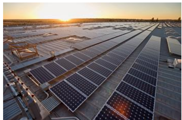
Photovoltaic (PV) solar array
