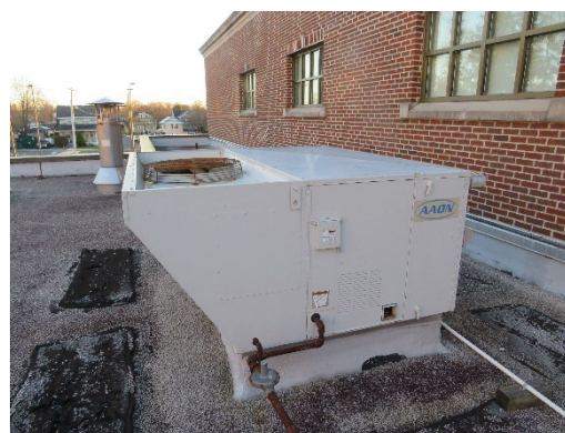
Walter Hill School - RTU
