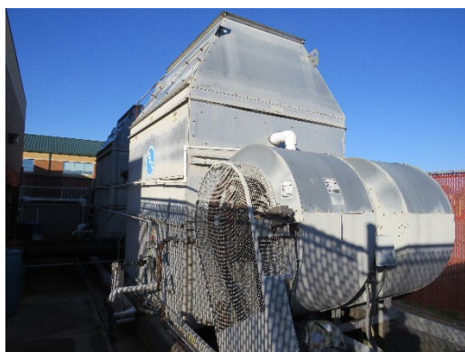
Governor Charles C. Stratton School – Cooling Tower
