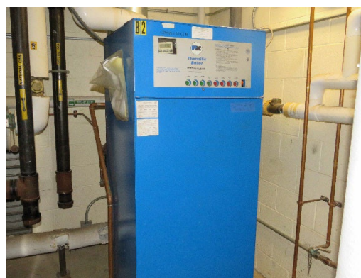
Margaret C. Clifford School - Boiler
