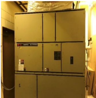
Image 2 AHU-1 Self-contained unit
