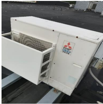
Image 11 Split system condensing unit
