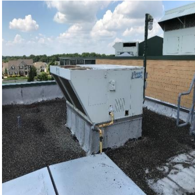
Image 8 Aeon RTU unit
