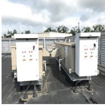
Image 9 AHUs on roof
