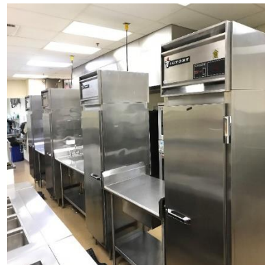
Image 27 Insulated heating cabinets
