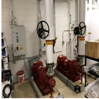
Image 13 Heating hot water pumps
