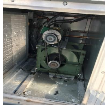
Image 10 Supply fan and motor
