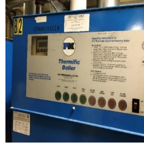
Image 6 Boiler plate information
