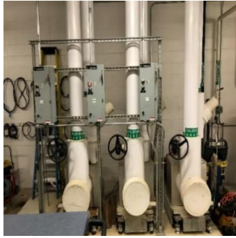
Image 19 Primary chilled water pumps
