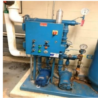
Image 16 Domestic cold-water pump
