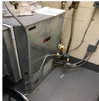
Image 3 Water source heat pump
