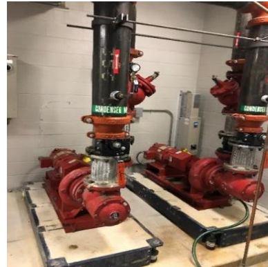
Image 15 Condenser water pumps
