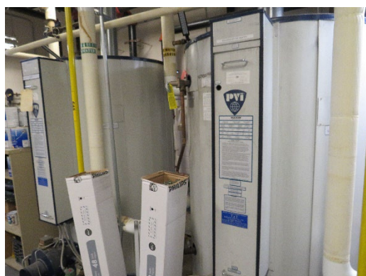
Governor Charles C. Stratton School – Water Heater
