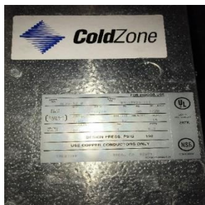
Image 23 Walk-in cooler nameplate
