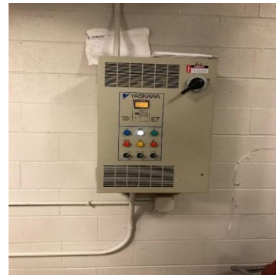
Image 17 VFD for HHWP pump
