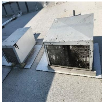
Image 29 Condensing unit on roof
