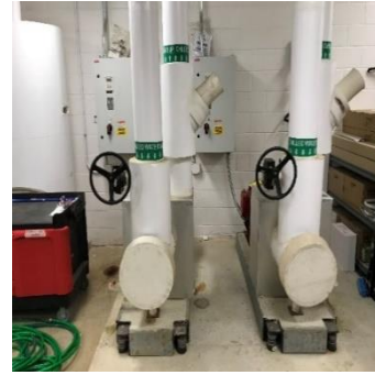
Image 20 Secondary chilled water pumps
