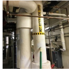
Image 8 Hot water supply pipe
