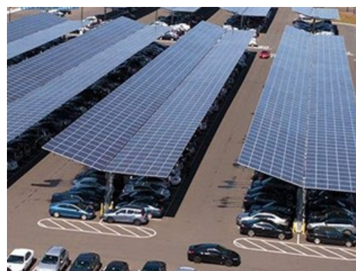
Typical Parking Lot Solar Array
