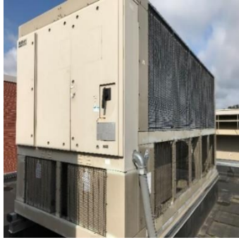
Image 17 Chiller 1 on roof
