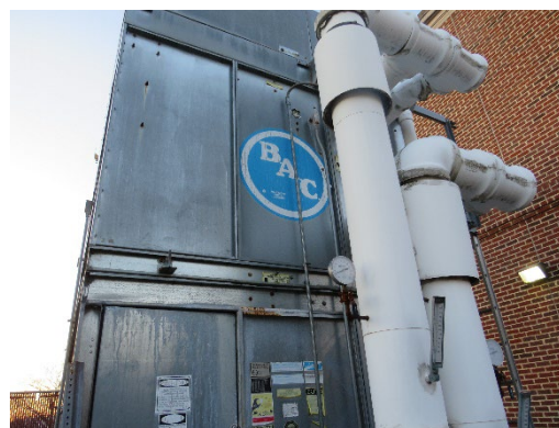
Walter Hill School – Cooling Tower
