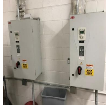
Image 14 VFDs for heating hot water pumps
