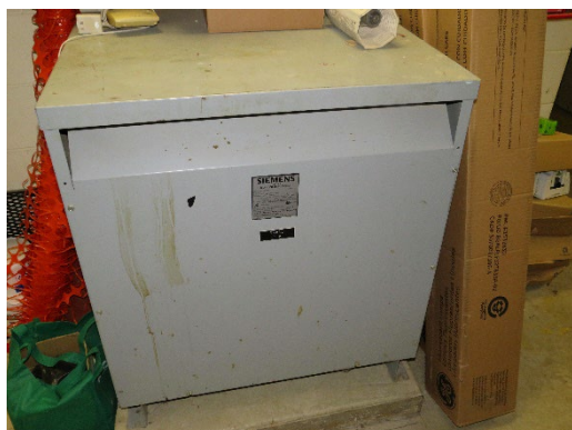
Margaret C. Clifford School - Transformer
