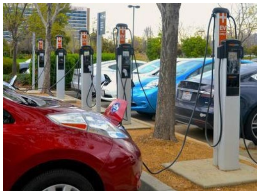
Sample Level 2 EV Chargers
