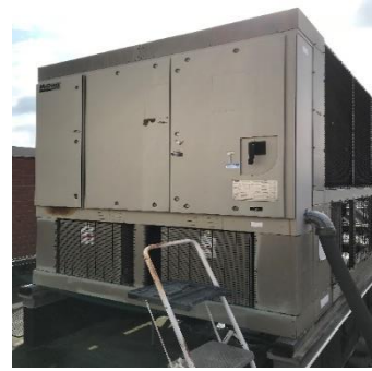
Image 18 Chiller 2 on roof
