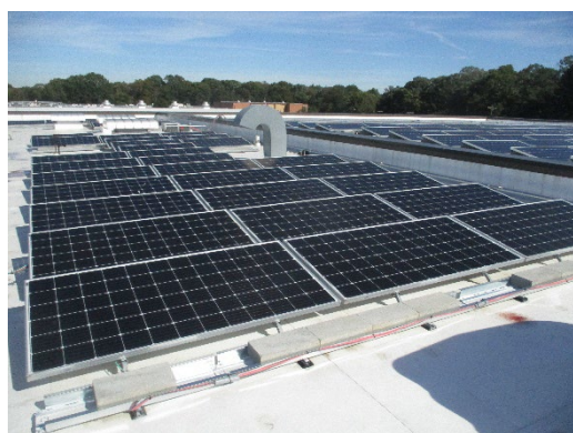
Typical Rooftop Solar Array
