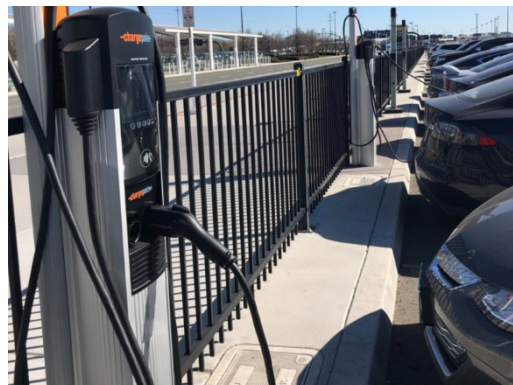
Sample Level 2 EV Chargers
