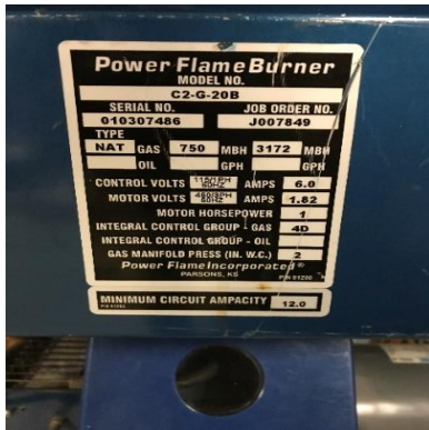
Image 14 Boiler burner nameplate
