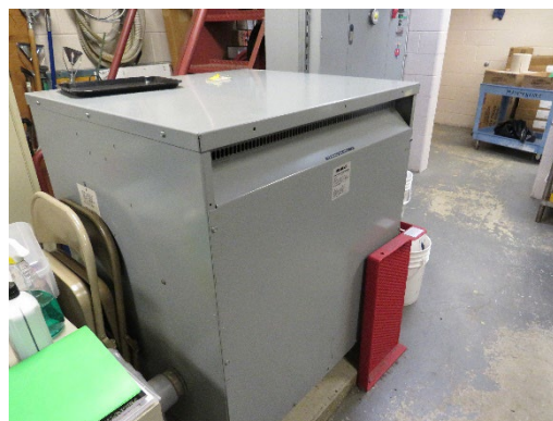
Governor Charles C. Stratton School - Transformer
