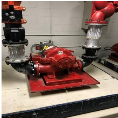
Image 16 Heating hot water pump
