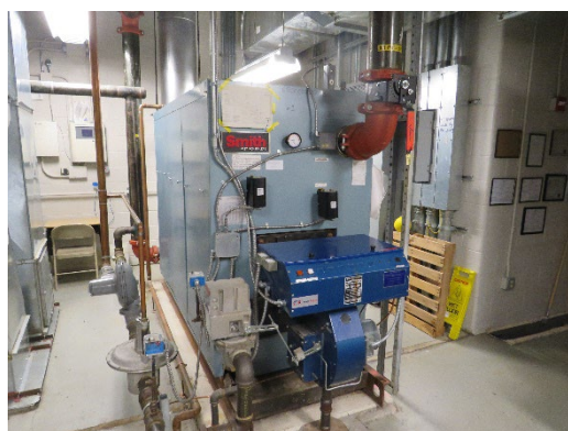
Governor Charles C. Stratton School - Boiler
