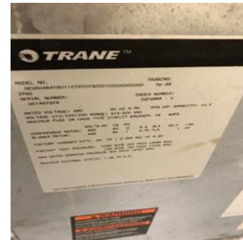
Image 4 Heat pump nameplate
