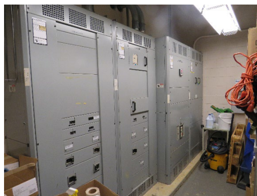
Governor Charles C. Stratton School – Switchboard
