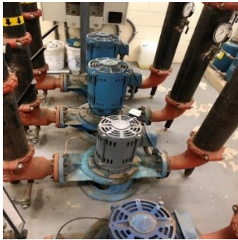
Image 15 Heating and condenser water pump
