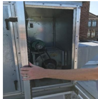
Image 12 Packaged unit interior
