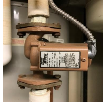
Image 22 Taco recirculation pump
