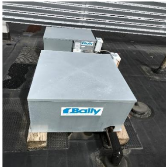
Image 33 Condensing units on roof
