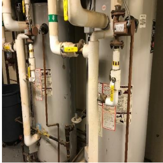
Image 21 Two hot water heaters
