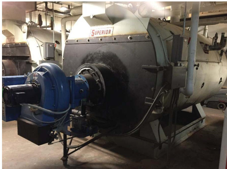
Figure 2: Wanaque ES Boiler Plant
