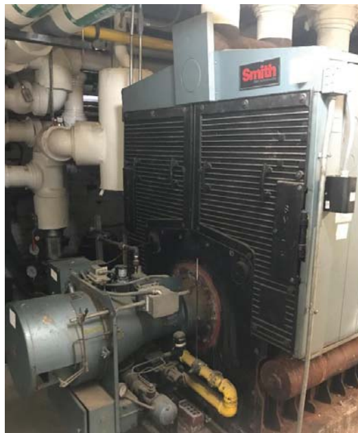
Figure 4: Haskell ES Boiler
