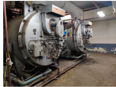
Figure 2.1: Existing Hot Water Boilers to be replaced Wayne Valley High School.
