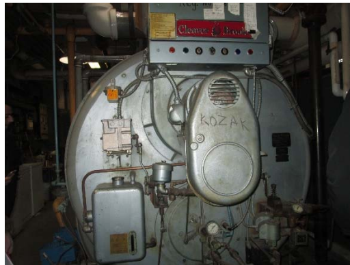
Boilers in Need of Burner Controls
