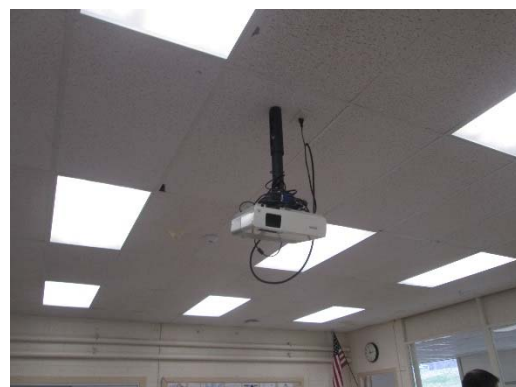
Examples of existing interior lighting
