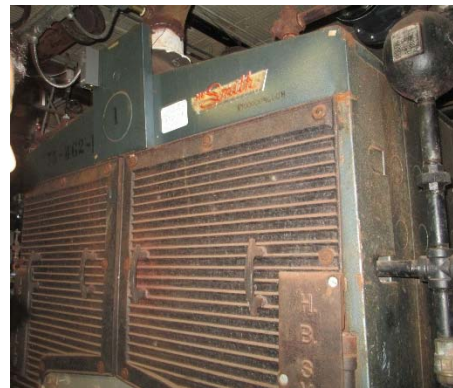
Existing Boilers to be Replaced
