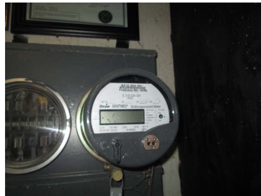
Existing Electrical Meters
