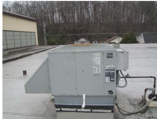
Existing Rooftop Units to be Replaced
