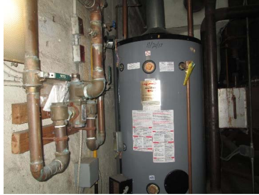
Examples of Uninsulated Piping
