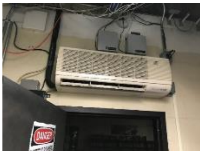
Split AC Unit
