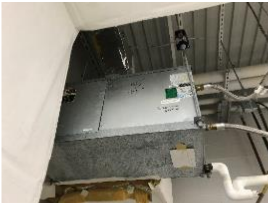
Water Source Heat Pump Unit
