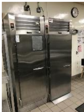
Reach -in Refrigerator
