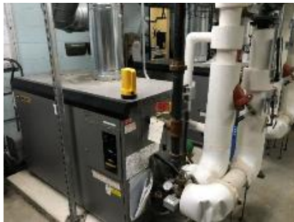
Condensing Hot Water Boiler
