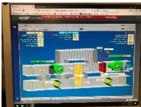
Heat Pump Unit
