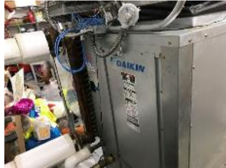
Water Source Heat Pump Unit
