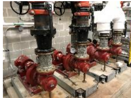
Heating Hot Water Pumps
