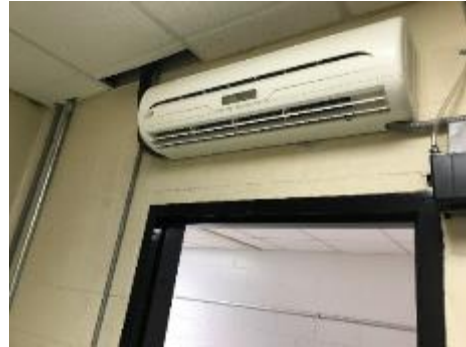
Split AC Unit
