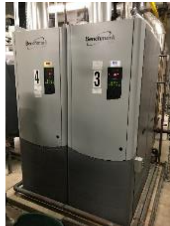
Condensing Hot Water Boilers
