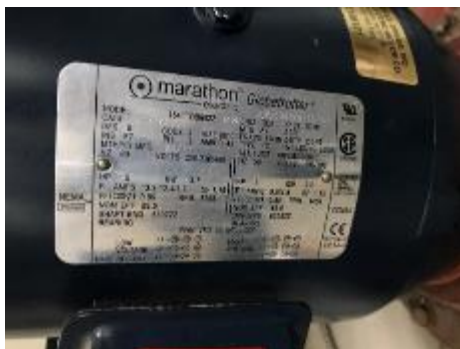
Heating Hot Water Pump
