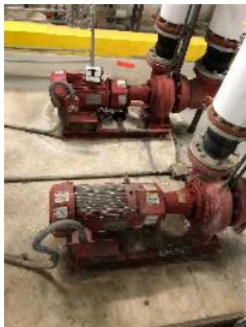
Heating Hot Water Pumps
