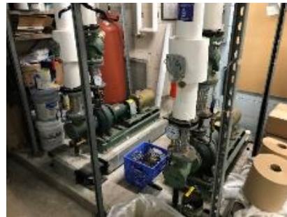
Heating Hot Water Pumps
