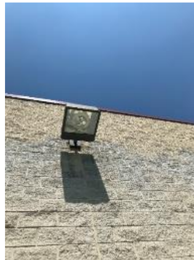
Wall-mounted LED Fixture
