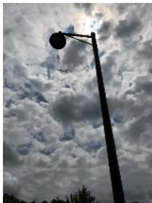
Pole-mounted Exterior Fixture
