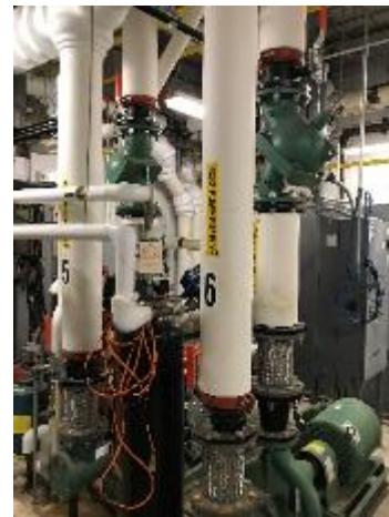
Heat Pump Supply Pumps
