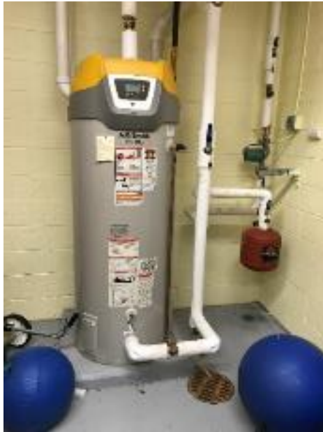
AO Smith Water Heater
