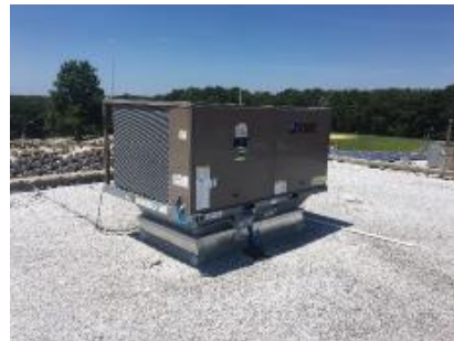
Cafeteria Packaged Units
