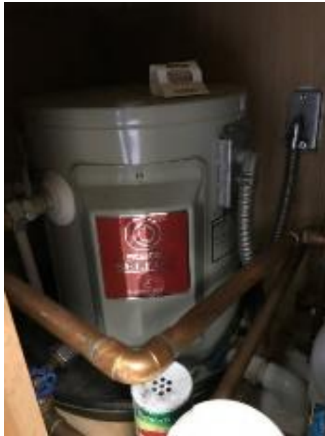
Hot Water Heater
