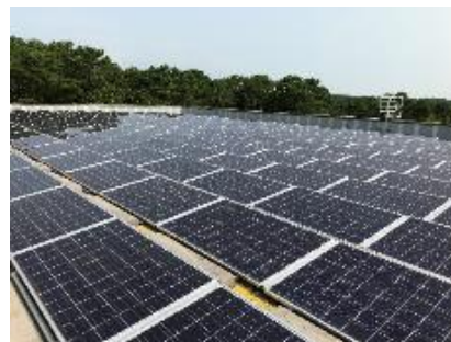
Solar Array (closeup)
