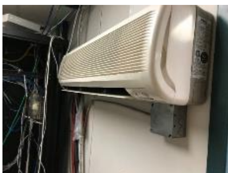
Split AC Unit
