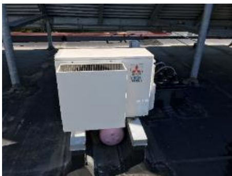
Split AC Unit
