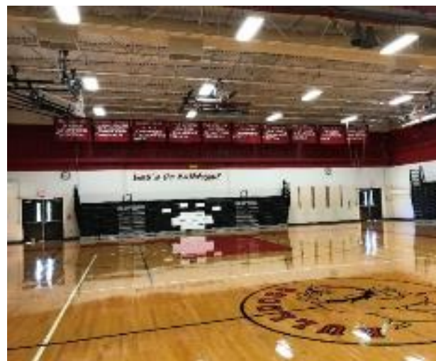
Gym Lighting T5 Fixture
