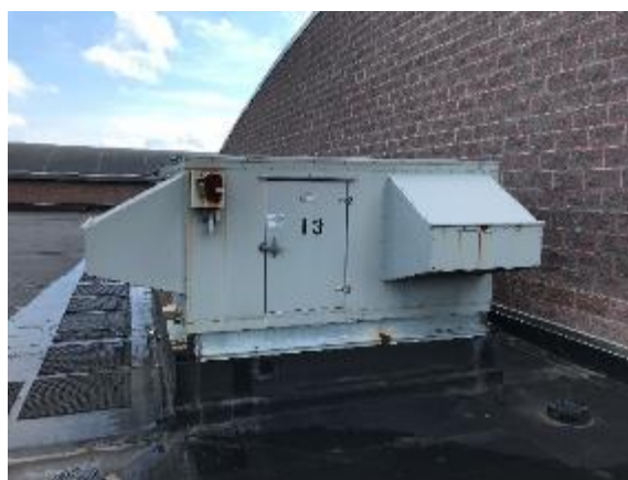
Air Handling Units
