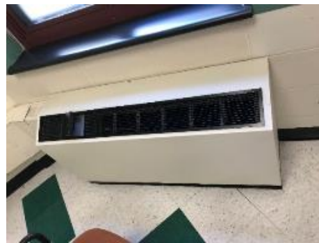
Heat Pump Unit
