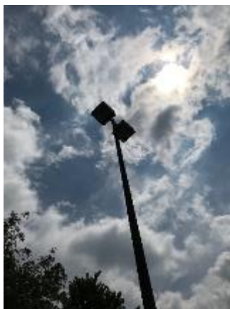
Exterior Pole Fixtures
