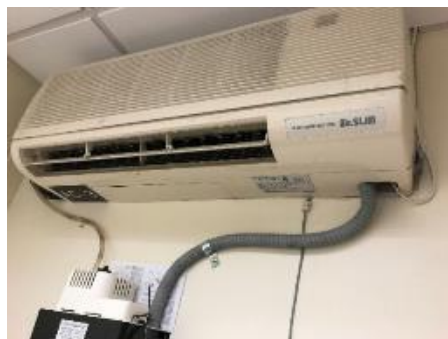
Split AC Unit
