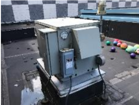
Energy Recovery Units
