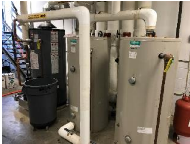
Hot Water Heater
