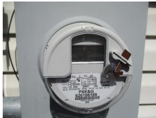
Load Reduction – Electric Meter at Bogota Board Office-Admin Building
