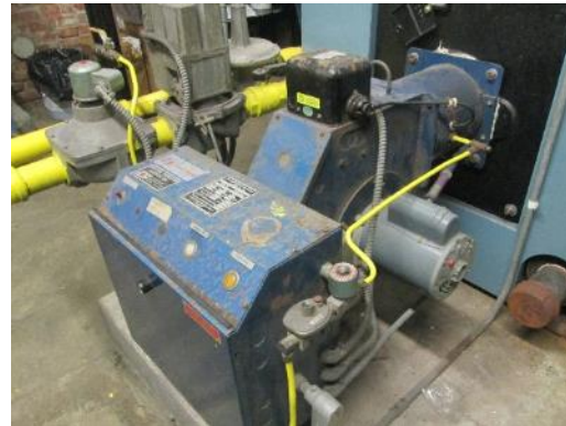
Burner Controls – Lillian M. Steen Elementary School
