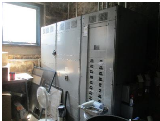
Load Reduction – Switchgear at Lillian M. Steen Elementary School
