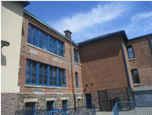
Existing Outdoor Lighting at Lillian M. Steen Elementary School
