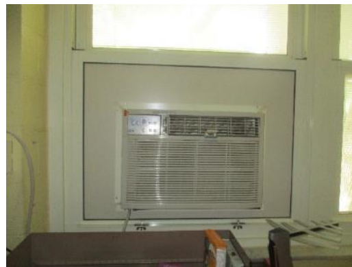
Window AC Unit – Bogota Jr. and Sr. High School
