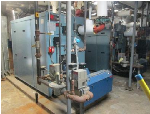
Burner Controls – E. Roy Bixby Elementary School
