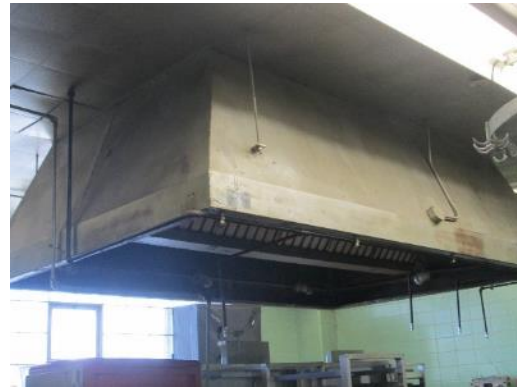
Kitchen Hood – Bogota Jr. and Sr. High School
