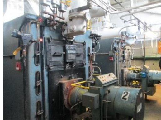
Boilers – Bogota Jr. and Sr. High School
