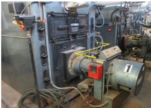
Boilers – Bogota Jr. and Sr. High School
