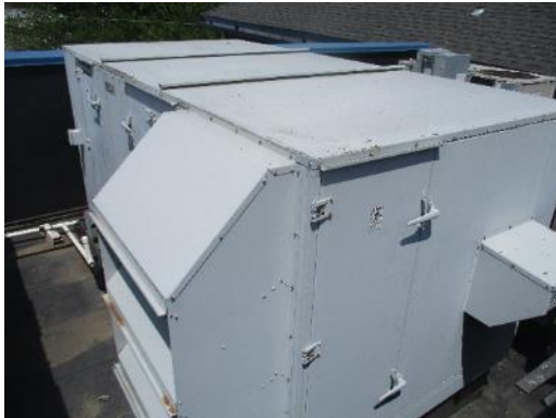
Existing Equipment – Lillian M. Steen Elementary School
