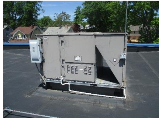
Existing Equipment – E. Roy Bixby Elementary School
