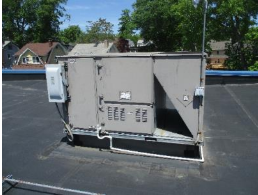
RTU – E. Roy Bixby Elementary School
