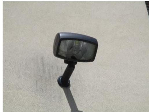
Existing Outdoor Fixture at Lillian M. Steen Elementary School
