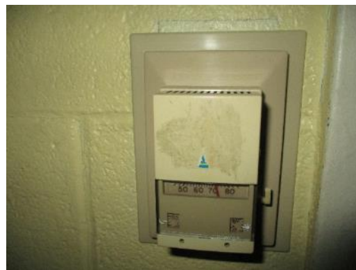
Existing Controls – Bogota Jr. and Sr. High School
