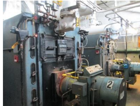
Boilers – Bogota Jr. and Sr. High School
