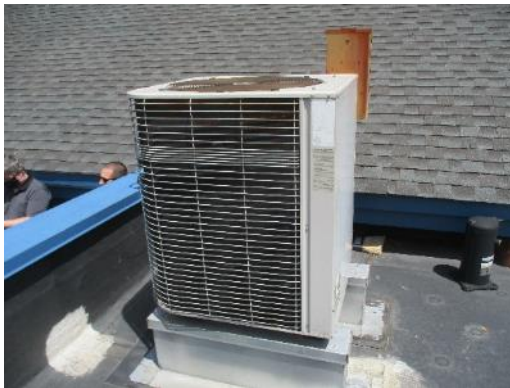
Split Unit – Lillian M. Steen Elementary School
