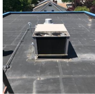
RTU – E. Roy Bixby Elementary School
