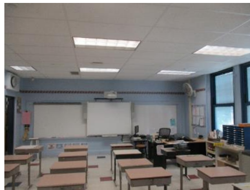
Lighting Control Space at E. Roy Bixby Elementary School
