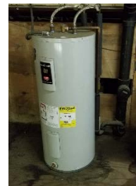
Domestic Hot Water
