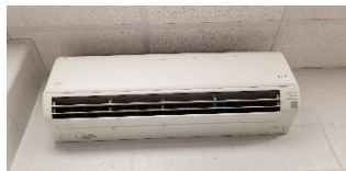
Split System AC (IT Room)
