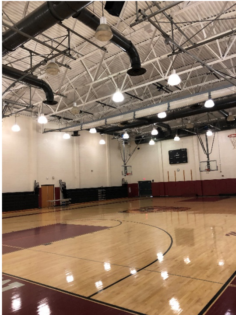
Memorial Middle School Light Fixtures
