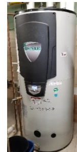
Domestic Hot Water
