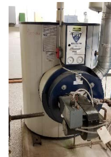
Domestic Hot Water
