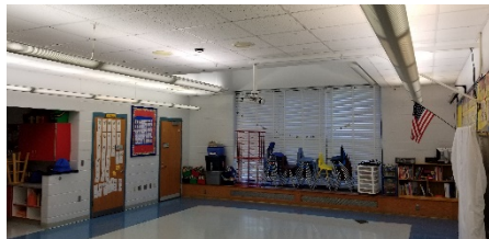
Typical Classroom Lights
