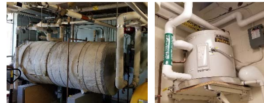
Domestic Hot Water
