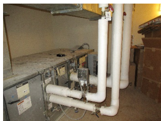
Air Handler Unit (AHU)
