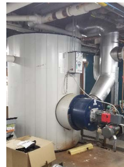
Domestic Hot Water
