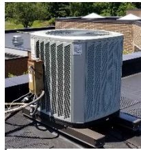
Split-System AC Condenser
