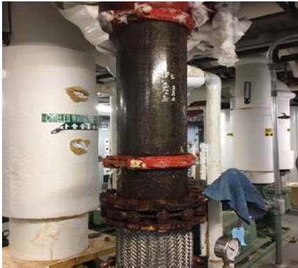
The un-insulated pipes (Memorial Middle)
