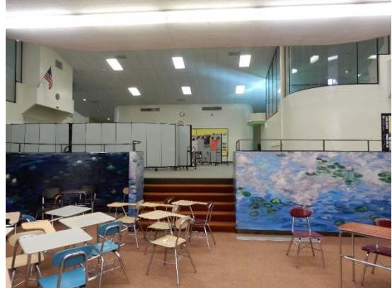
Figure 7. Open Classroom with Unit Ventilator Grilles
