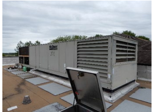
Figure 9. Section 700/800 Rooftop Unit (RTU)
