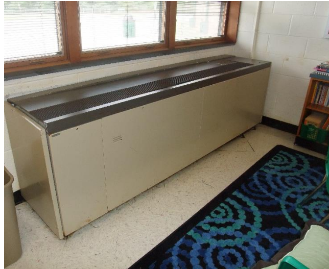
Water Source Heat Pump Unit
