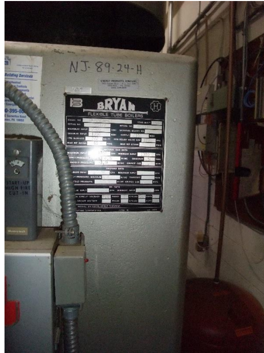
Hot Water Boiler
