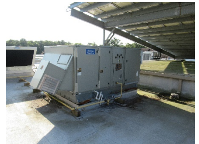
One of the three RTUs currently using R22 refrigerant to be retrofit
