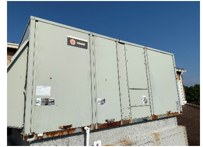
One of the two TRANE RTUs serving the Gym to be Replaced
