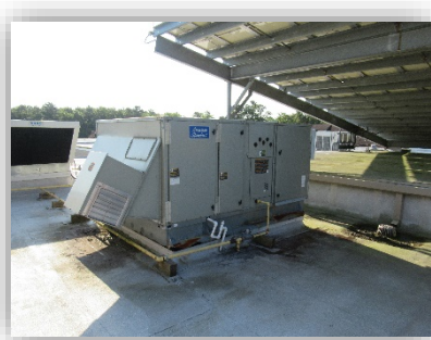
Media Center RTU at Frog Pond Elementary
