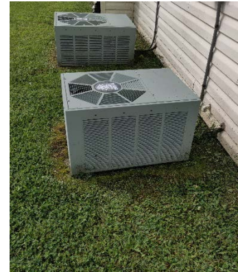
Typical AC Units Outside of BOE Offices
