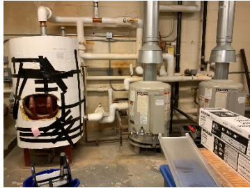
Domestic Hot Water
