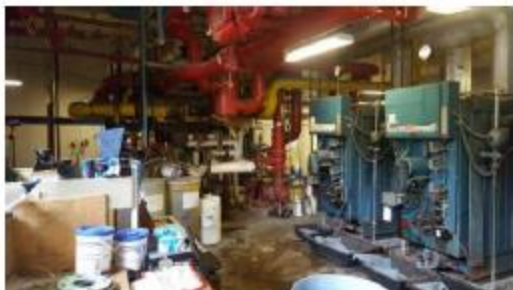
Pipe Insulation – boiler room #1 is proposed to undergo a full heating distribution retrofit. There are no recommendations to complete pipe insulation measures in this room with the exception of a small amount of work in the domestic hot water system.
