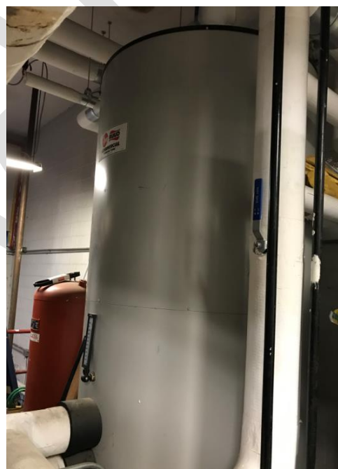
Figure 9A.2 – Existing DHW Heater tank
