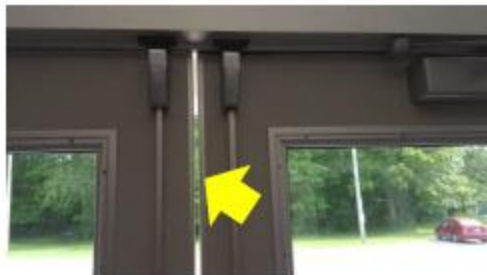
Door Weather Stripping – daylight visible at the center of the door is a clear indicator of an unwanted air leakage pathway due to missing weather stripping materials.
