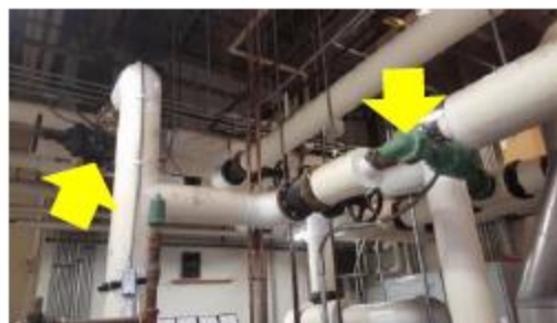
Pipe Insulation – heating distribution pipes are mostly insulated. Select flanges, valves, and fittings that were left bare need to be insulated.
