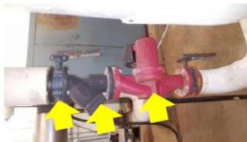
Valve & Fitting Insulation – butterfly valves, strainers, and pumps pictured above require insulation to avoid distribution losses.
