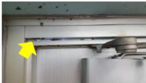
Caulking – weather stripping installed to the snap trim is useless when air is allowed to bypass snap trim into the building. Caulking the snap trim in place eliminates air leakage pathways around the door in turn allowing weather stripping to create an effective air barrier.
