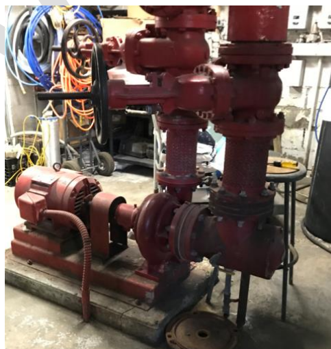
Figure 10.2 – Existing HHW Pumps
