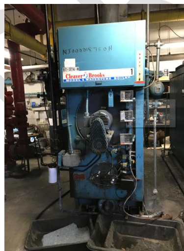
Figure 10.1 – Existing Cleaver Brooks Boiler
