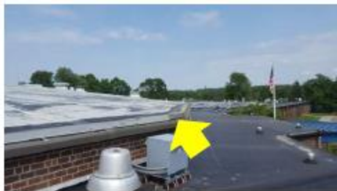
Roof-Wall Intersection Air Sealing – the exterior flashing and finishes at the roof-wall intersection are not constructed to stop air leakage; the elevation change at the Library/Media Center, Auditorium, and adjoining offices creates a construction detail susceptible to large amounts of air leakage.
