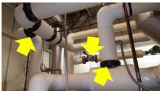
Pipe Insulation – heating distribution pipes are mostly insulated. Select flanges, valves, and fittings that were left bare need to be insulated.
