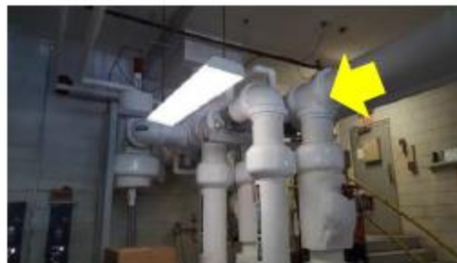
Pipe Insulation – chilled water pipe insulation was properly installed, there are no recommendations to wrap chilled water distribution pipes.
