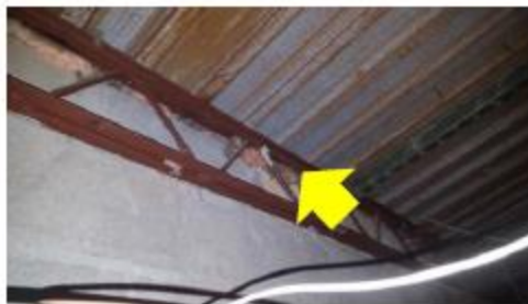
Roof-Wall Intersection Air Sealing – gaps at the interior of the roof-wall intersection combine with the unsealed exterior flashing and finish details to allow unwanted infiltration/ exfiltration; excessive debris and cobwebs collecting at the roof-wall are clear indicators of air leakage.
