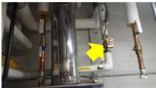
Valve & Fitting Insulation – the inline pump needs to be insulated in order to avoid unnecessary domestic hot water distribution losses.
