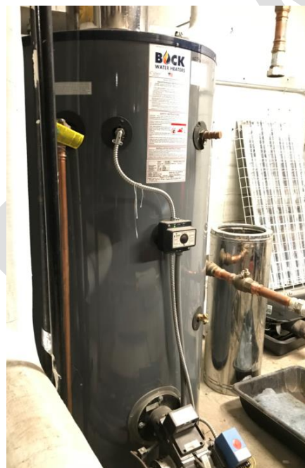
Figure 9A.1 – Existing DHW Heater
