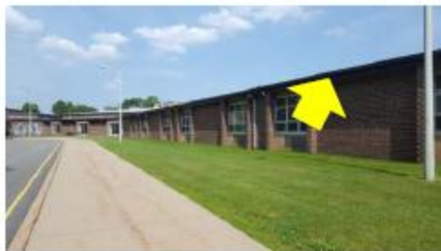
Roof-Wall Intersection Air Sealing – the exterior flashing and finishes at the roof-wall intersection are not constructed to stop air leakage.
