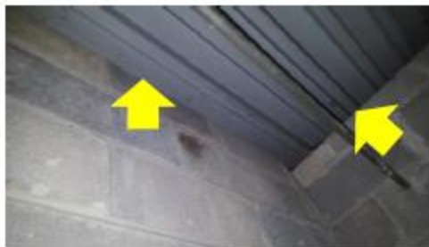
Roof-Wall Intersection Air Sealing – gaps at the roof and unsealed gaps around framing components create pathways for unwanted infiltration/ exfiltration; bypasses in the masonry components are allowing infiltration/ exfiltration.
