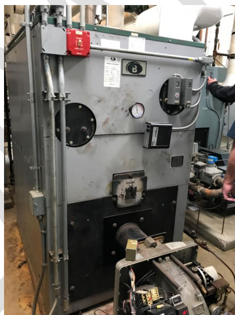
Figure 9.1 – Existing Boiler for E-Wing
