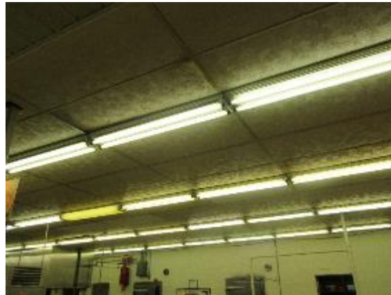
Macopin Middle School Lighting
