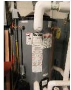
Domestic Hot Water
