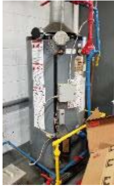
Domestic Hot Water
