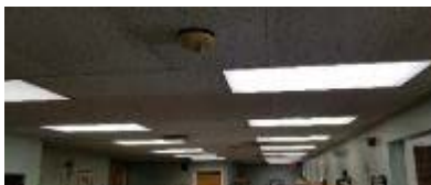
Administration Building Lighting
