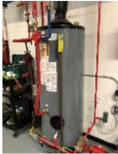
Domestic Hot Water
