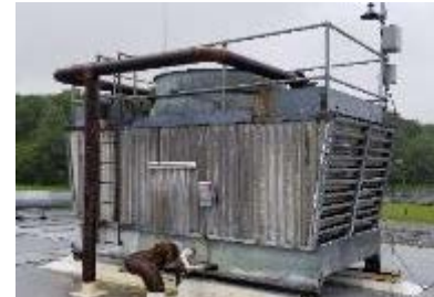
High School Cooling Tower
