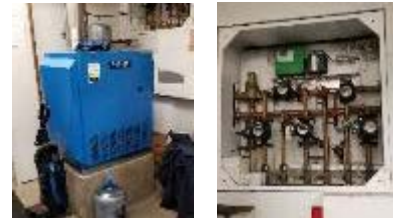
Hot Water Heating System
