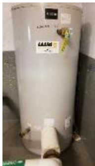
Domestic Hot Water
