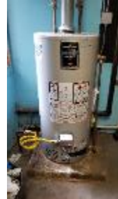
Domestic Hot Water
