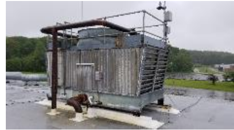
Chiller Water (CHW) Cooling Tower
