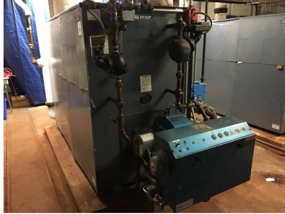
Existing burner at Vetter Elementary
