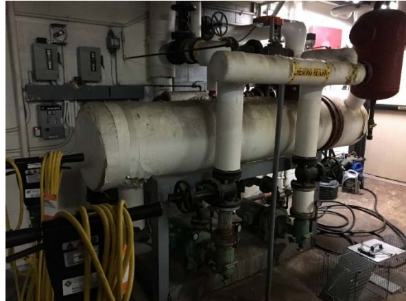
Existing Heat Exchanger at Vetter Elementary
