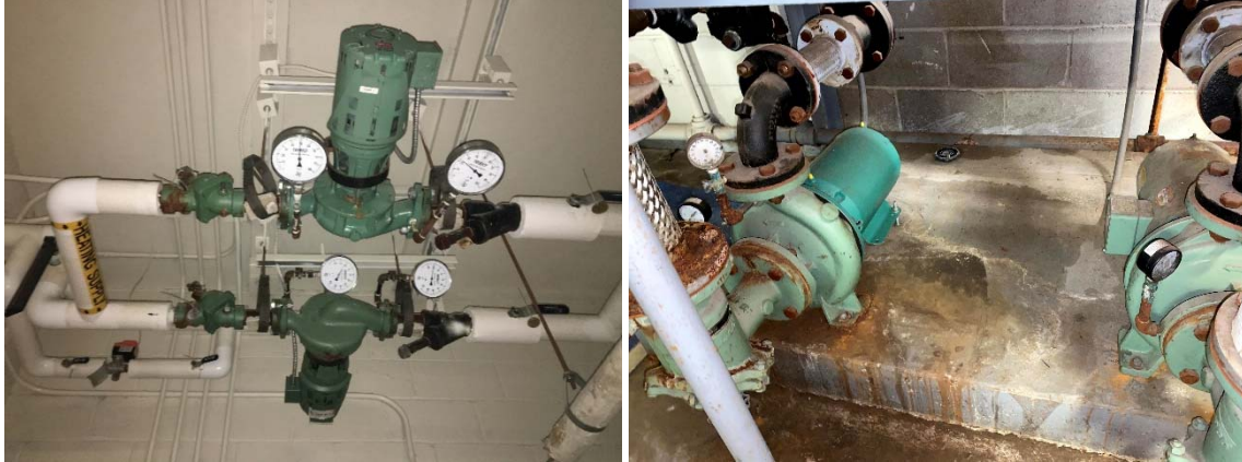
Existing Hot Water Loop Pumps at Vetter Elementary
