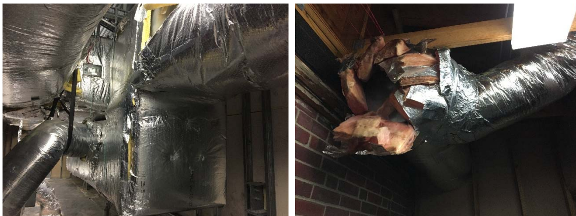
Existing ductwork at Memorial Middle School and Vetter Elementary
