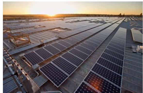
Photovoltaic (PV) solar array
