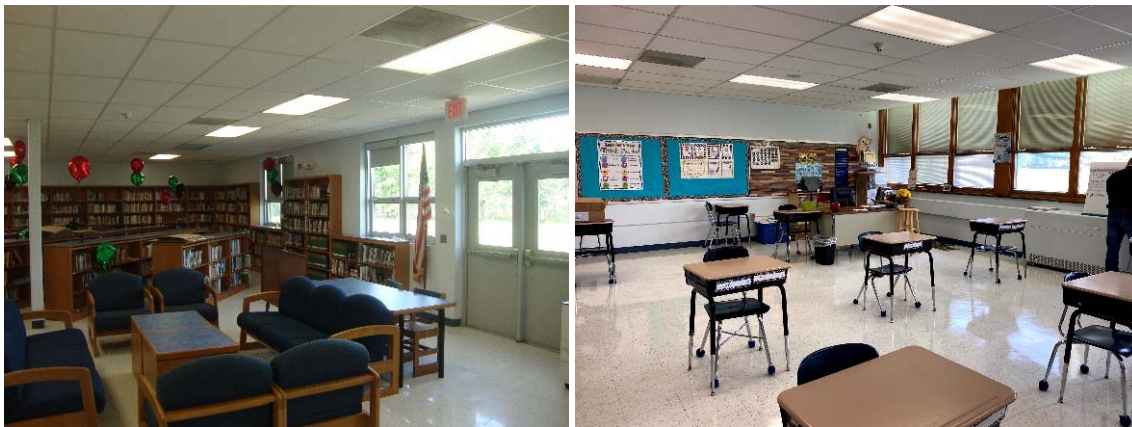
Existing interior lighting at Memorial Middle School and Margaret L Vetter Elementary
