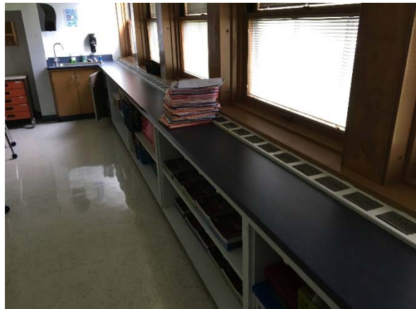
Existing baseboard in steam loop classroom
