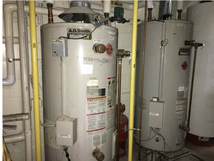
Existing Hot Water Heater Tanks at Memorial Middle School
