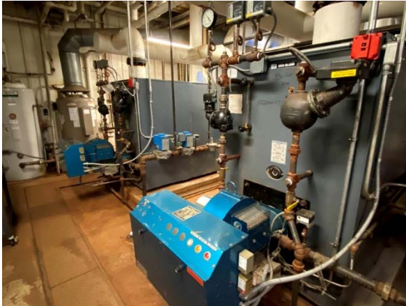
Existing Steam Boilers at Vetter Elementary
