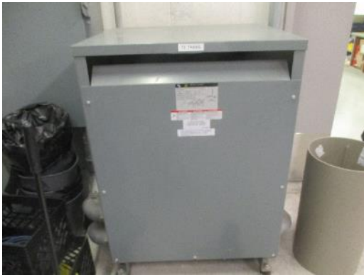
Transformer – Marti School 28
