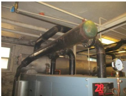
Boiler Piping – Ben Franklin School - 13
