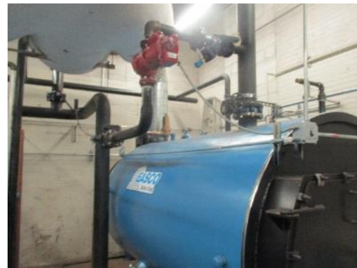
Boiler Piping - Lafayette School - 6
