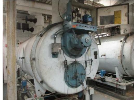
Boilers – Washington/Dunn Academy 1
