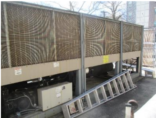
Chiller – Battin McAuliffe School 4
