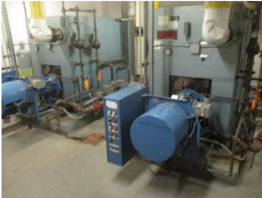
Boilers – Sonia Sotomayor School 25
