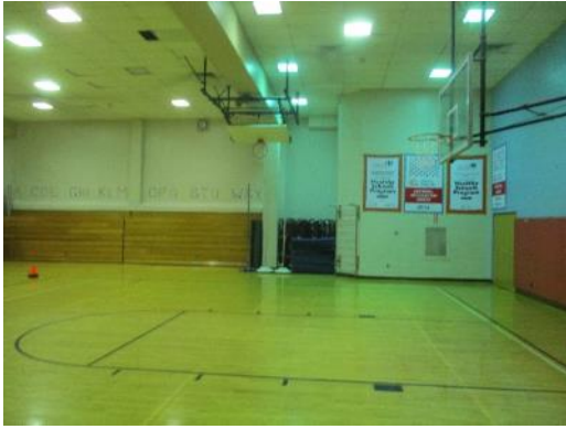
Lighting at La Corte-Peterstown School 3
