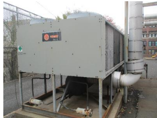
Chiller – Terence C. Reilly School 7
