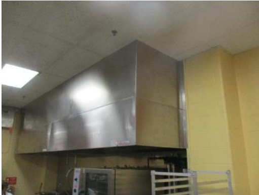
Kitchen Hood –School 30
