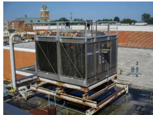
Cooling Tower – Washington School 1
