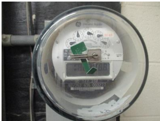
Load Reduction Electric Meter
