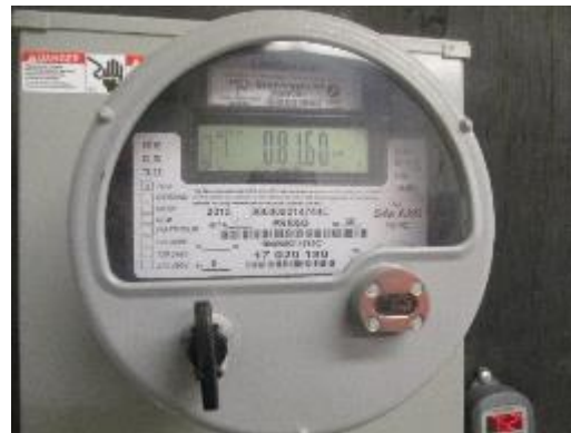
Load Reduction – Electric Meter
