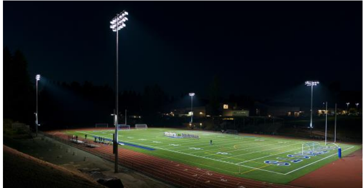
Example of Stadium Lighting
