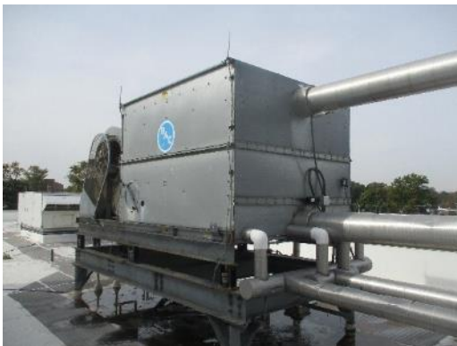
Cooling Tower – Dr. A. Pantoja School 27
