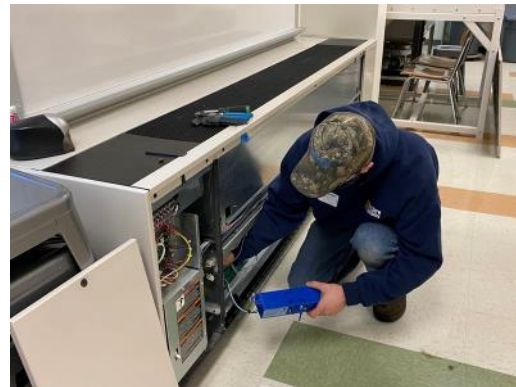
NPBI and Controls – Installed in Classroom Unit Ventilator
