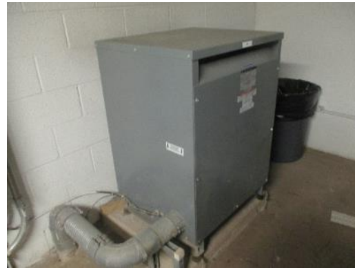
Transformer – Edreira School 26
