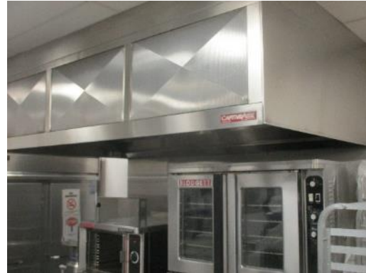
Kitchen Hood –School 81
