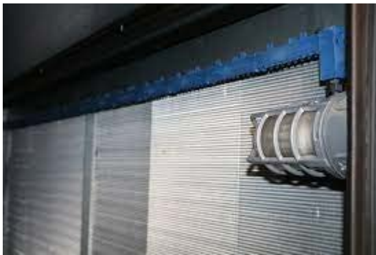
NPBI – Installed in Typical AHU Coil
