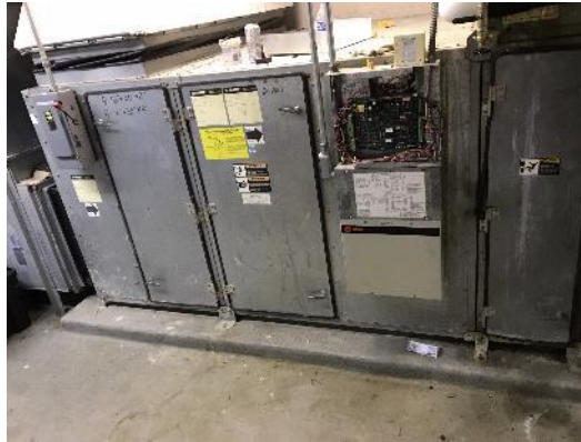
Figure 5: AHU-2 serving B-5 Housing
