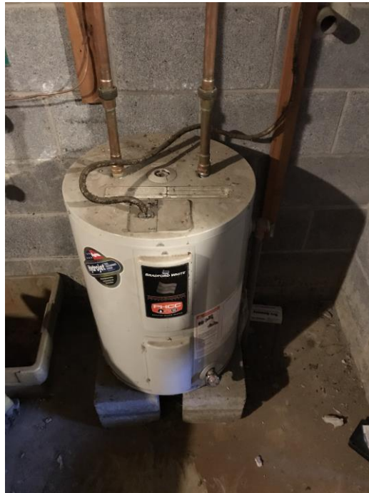
Figure 3: DHW Water Heater
