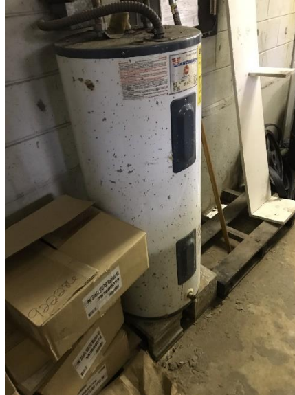
Figure 7: DHW-1 Boiler Room
