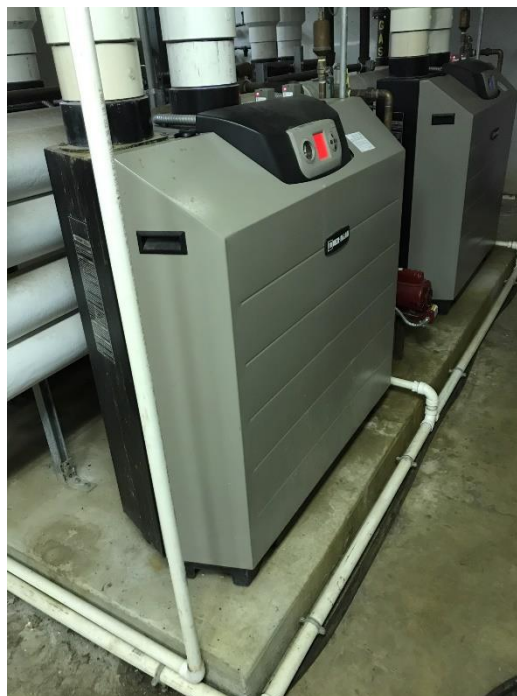
Figure 2: Two (2) 750 MBH Gas-Fired Boilers
