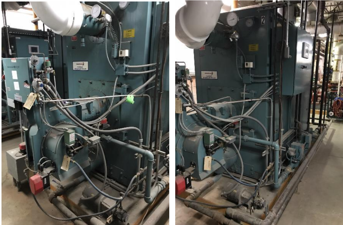
Figure 2: Two (2) 6,00 MBH Input Gas-Fired Boilers
