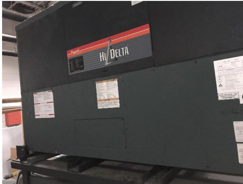
Figure 7: DHW-1 Boiler Room
