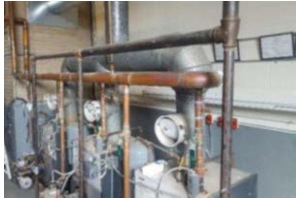
Uninsulated Pipes (High School)
