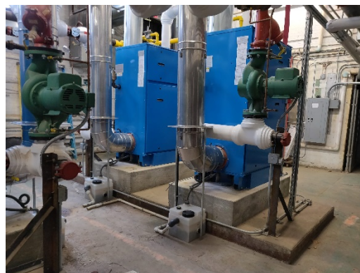
Figure 6 Asbury Park High School Boilers
