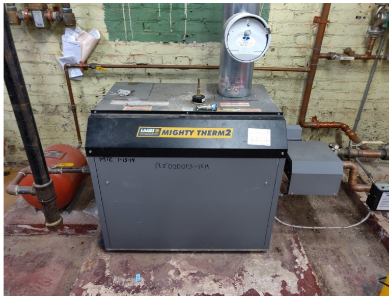
Figure 18 Barack Obama ES Domestic Hot Water Heater
