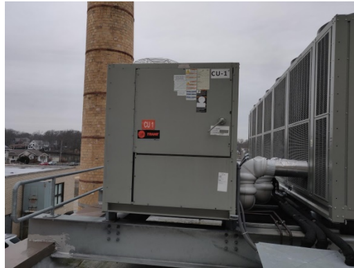
Figure 4 Asbury Park High School Air Handling Unit (Rooftop)
