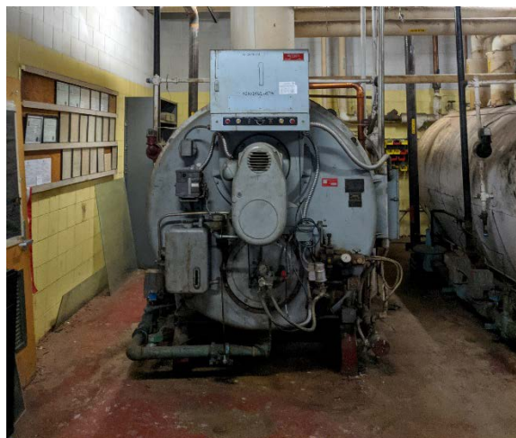
Figure 11 MLK Jr. MS Boiler
