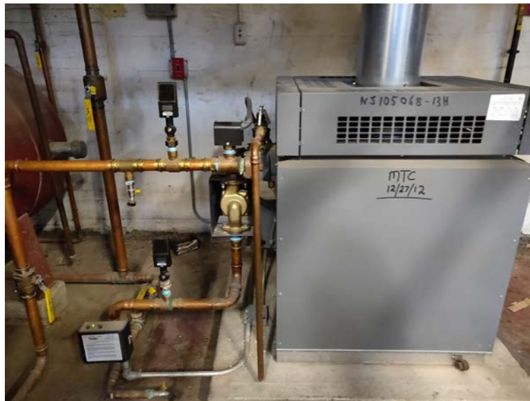
Figure 8 Asbury Park High School Domestic Hot Water Heater
