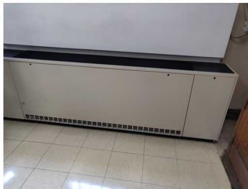
Figure 7 Asbury Park High School Classroom Unit Ventilator
