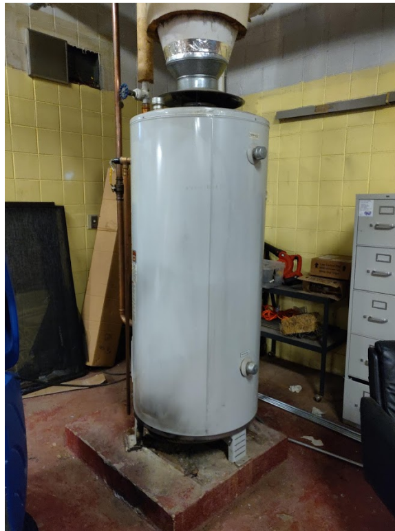
Figure 12 MLK Jr. MS Domestic How Water Heater
