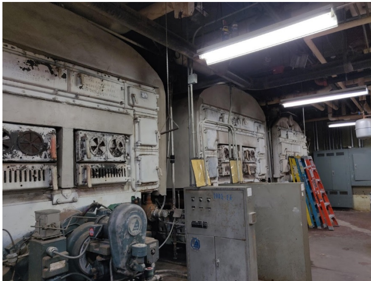
Figure 17 Barack Obama ES Boilers
