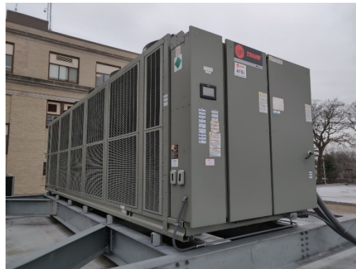
Figure 5 Asbury Park High School Air Cooled Chiller
