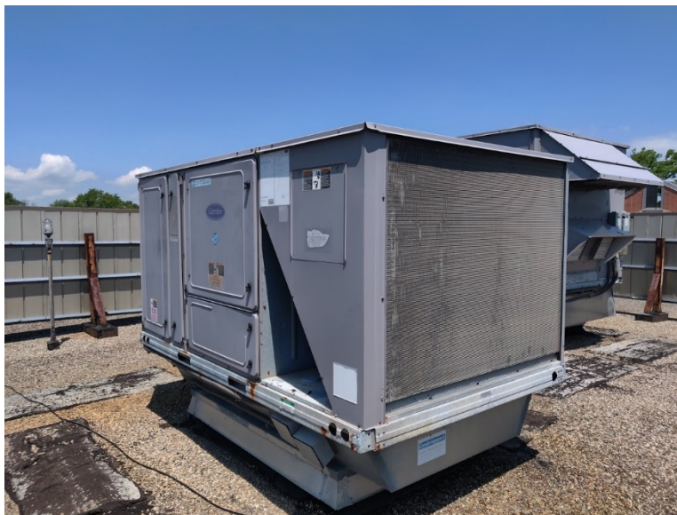
Figure 14 Bradley ES Rooftop Unit
