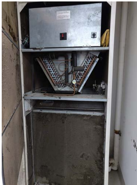
Figure 15 Bradley ES Classroom Unit Ventilator
