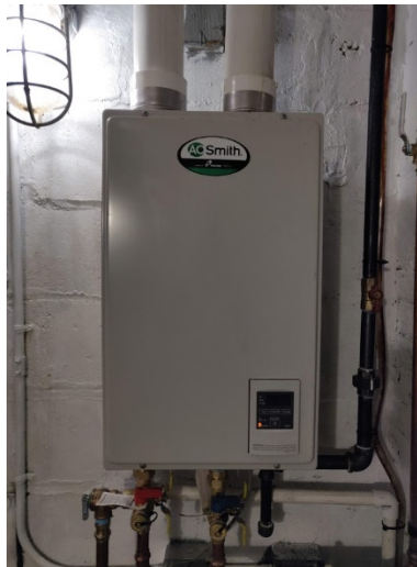
Figure 28 IT Center Domestic Hot Water Heater
