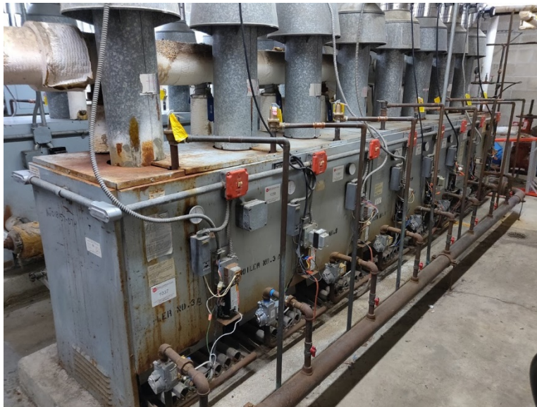
Figure 20 Thurgood Marshall ES Boilers
