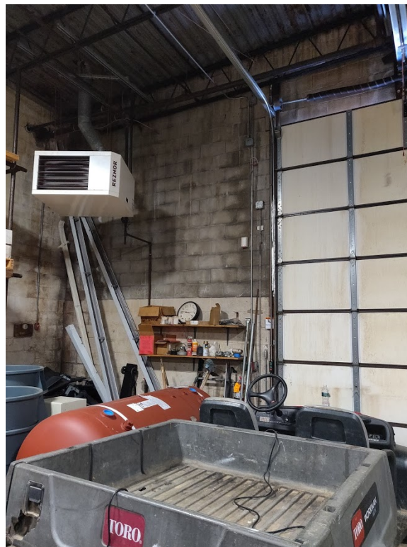
Figure 23 Buildings and Ground Ceiling Mounted Heater
