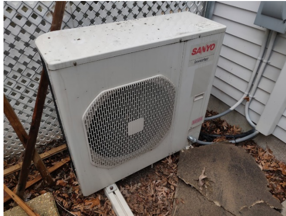
Figure 26 IT Center Split System AC
