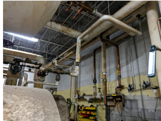
Uninsulated Pipes (Middle School)
