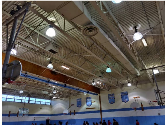
Figure 10 MLK Jr. MS Gym Lighting
