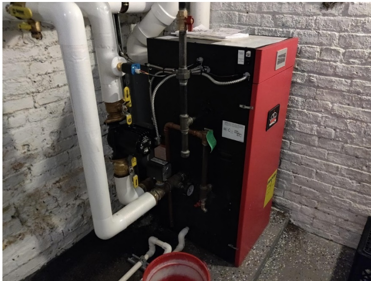
Figure 25 IT Center Boiler
