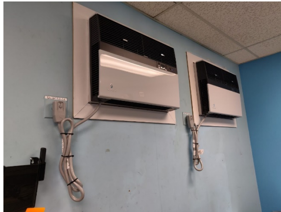
Figure 27 IT Center Through-Wall AC
