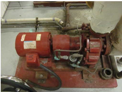
200 Wing Hot Water Pump – Sparta HS
