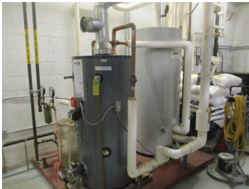
Domestic Water Heater – Sparta MS
