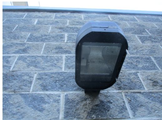
Existing Wall Lighting at Sparta MS
