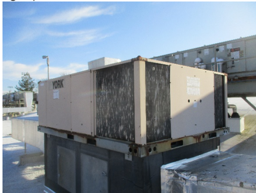
Roof Top Unit – Sparta HS
