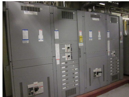
Sparta HS Electrical Panel
