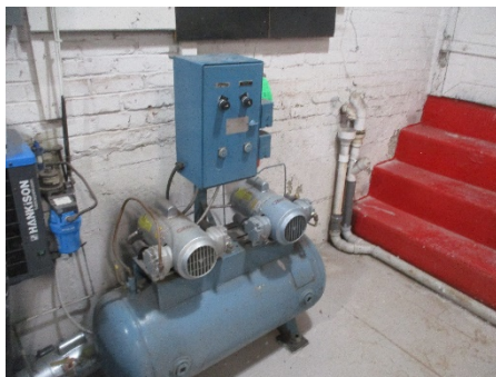
Pneumatic Controls – Mohawk ES
