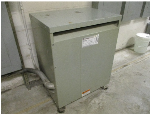
Transformer – Sparta MS
