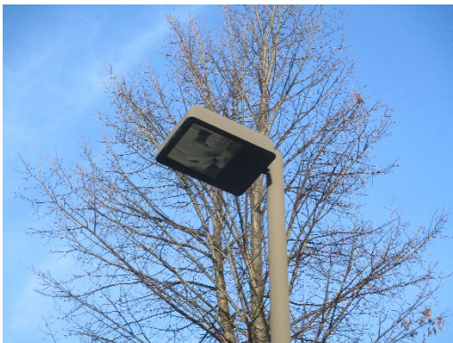
Existing Outdoor Lighting at Sparta MS
