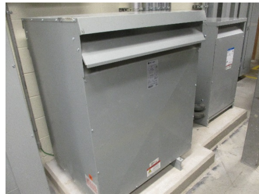
Transformer – Sparta HS
