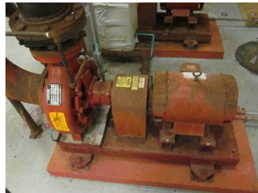
200 Wing Cooling Tower Pump - Sparta HS
