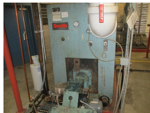
Boilers to Replace – Sparta HS
