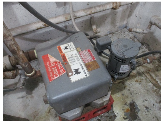
Mohawk Avenue School Steam System
