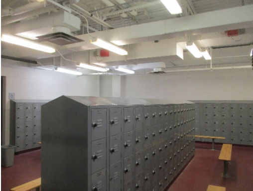
Existing Lighting at Sparta MS
