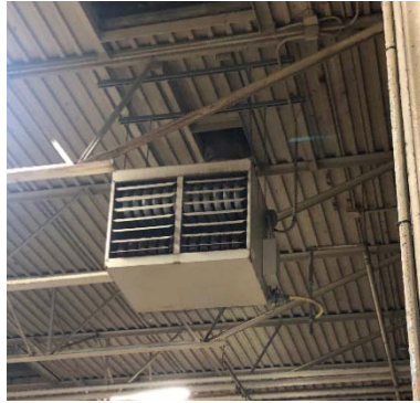
Existing unit heater at Ventnor Public Works
