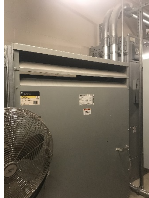
Existing transformer at Ventnor Educational Community Complex
