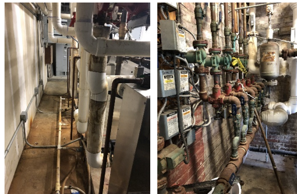
Damaged pipe and valve insulation at Ventnor Cultural Center and Ventnor Fire House 1
