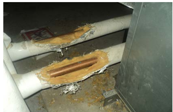
Uninsulated hot water piping
