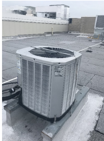
Existing split system condensing unit at Ventnor Educational Community Complex
