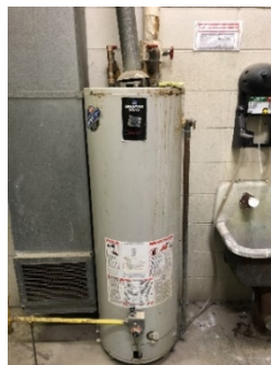
Existing domestic water heater at Ventnor Public Works
