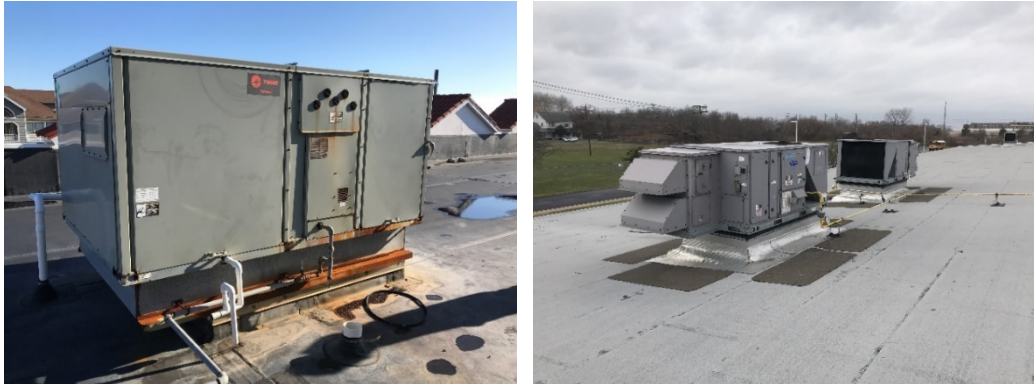
Existing roof top units at Ventnor Cultural Arts/Senior Center and Ventnor Educational Community Complex
