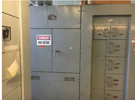
High School Electrical Service
