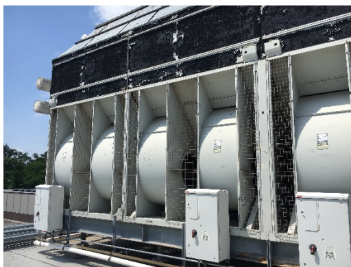
Cooling tower at Piscataway HS
