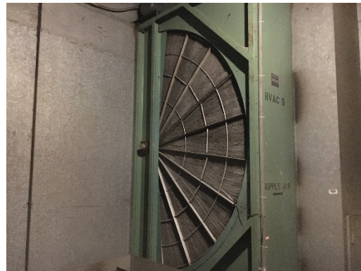
Energy Recovery Wheel at High School
