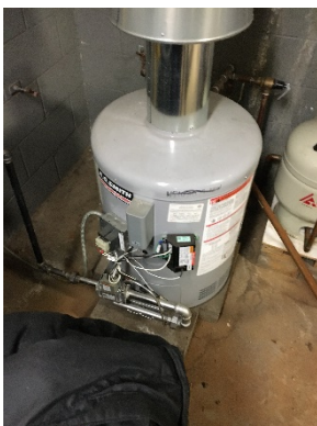
Water Heater at Quibbletown MS
