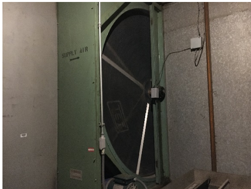
Energy Recovery Wheel at High School
