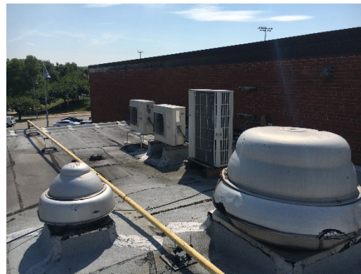
Exhaust Fans at Piscataway HS
