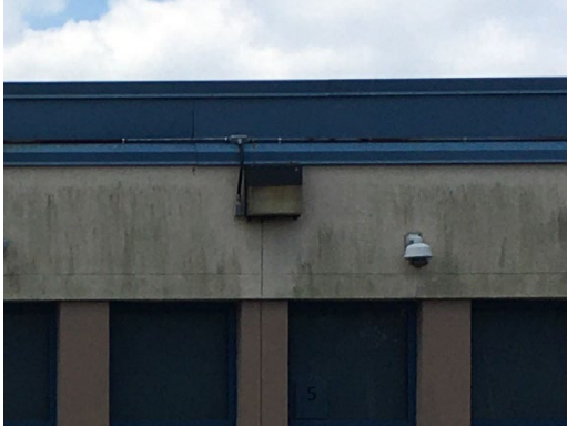
Existing Wallpack at Quibbletown MS
