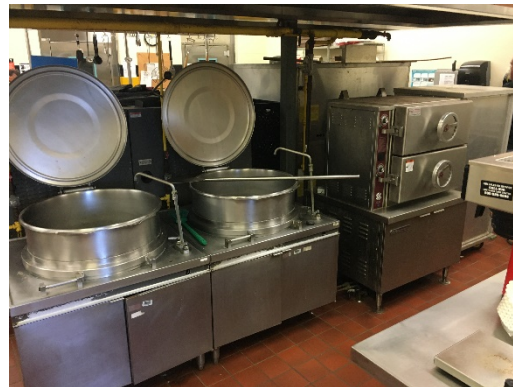
Central Kitchen Cooking Equipment
