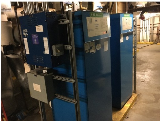
Boilers at Piscataway HS
