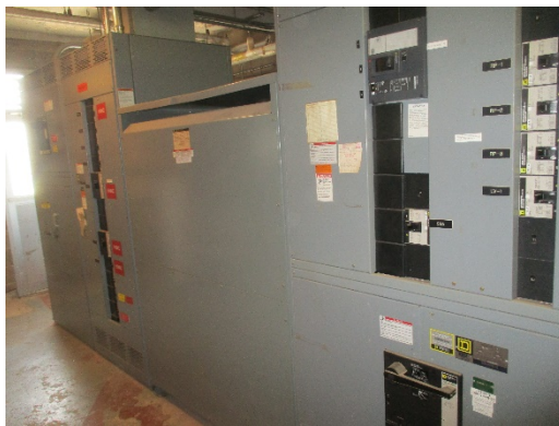
Electrical Service at Conackmack MS
