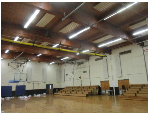
Lighting Control Space at Grandview
