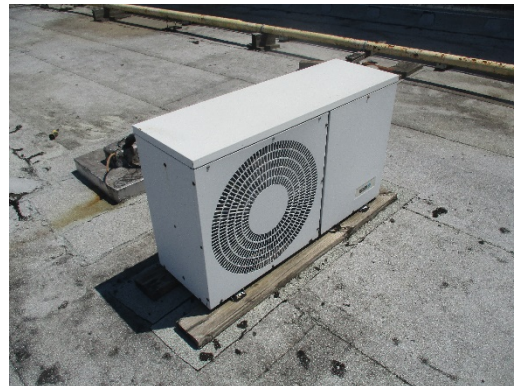
Split System Unit at Conackamack MS
