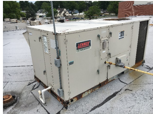
Rooftop Unit at Arbor IS
