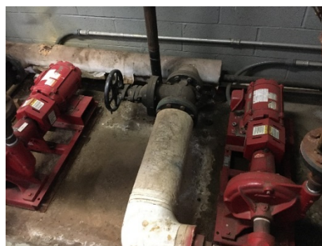
Pump Motors at Quibbletown MS
