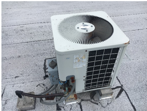
Split System Unit at Randolphville ES
