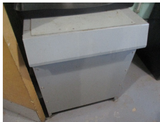
Transformer at Arbor IS
