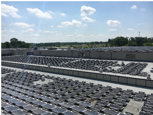
Rooftop Solar Array
