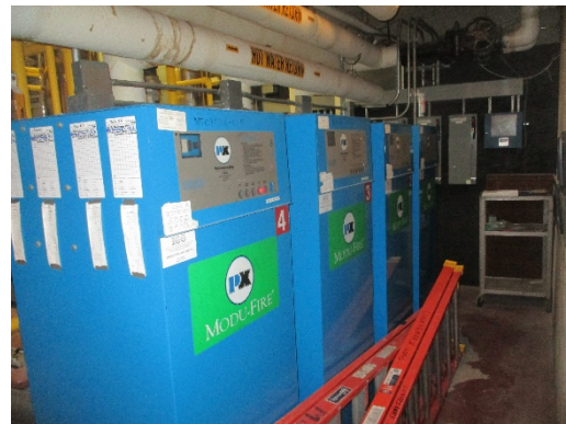
Boilers at Conackamack MS
