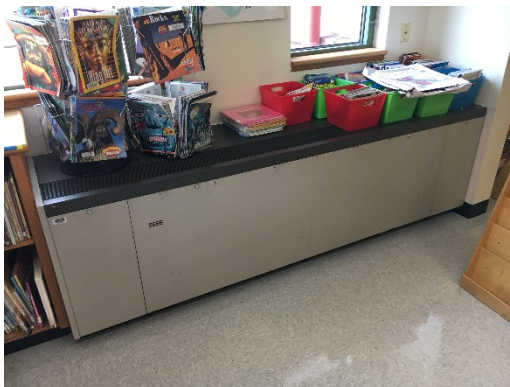
Unit Ventilator at Randolphville ES
