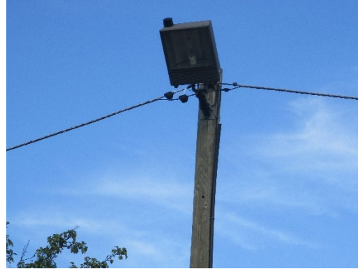
Existing Pole Light at Grandview ES
