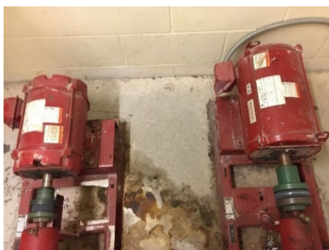
Pump Motors at Piscataway HS
