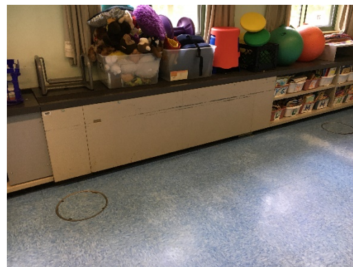
Unit Ventilator at Knollwood ES
