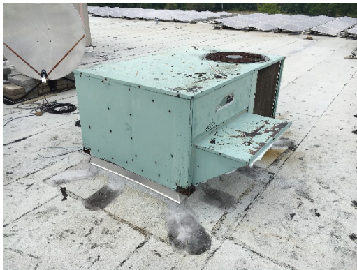
Rooftop Unit at Piscataway HS
