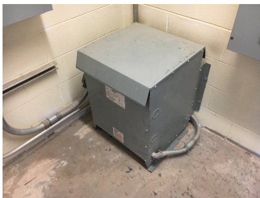
Transformer at Piscataway HS
