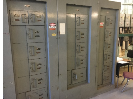
High School Electrical Service
