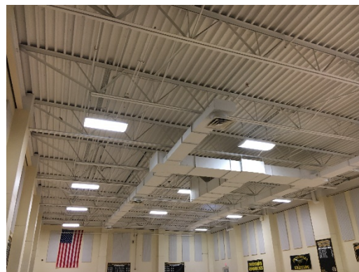
Lighting Control Space at Piscataway HS
