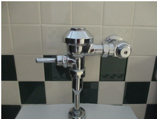
Flush Valve at Arbor IS
