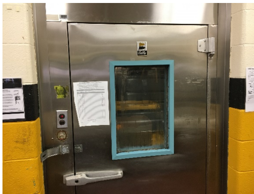
Walk-in Cooler at Piscataway HS
