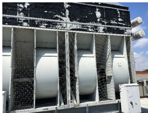
Cooling tower at Piscataway HS
