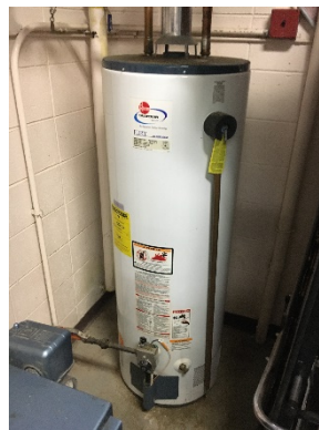
Water Heater at Randolphville ES
