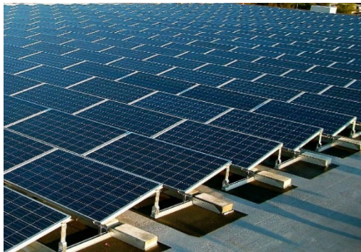
Rooftop Solar Array
