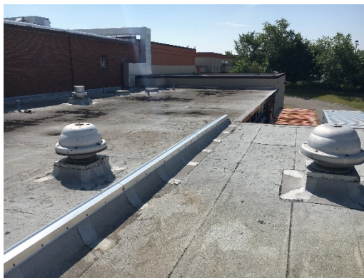
Exhaust Fans at Piscataway HS
