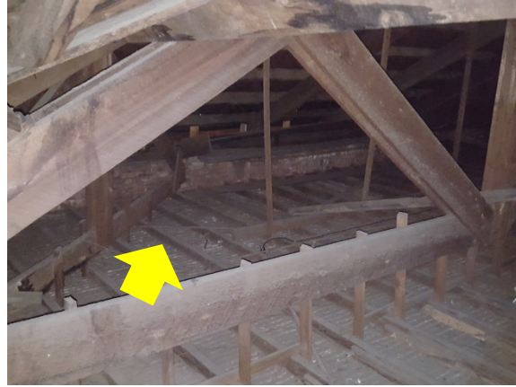
Attic Bypass Air Sealing & Insulation –no insulation at the attic flat for controlling heat loss or heat gain (Benjamin Franklin School).
