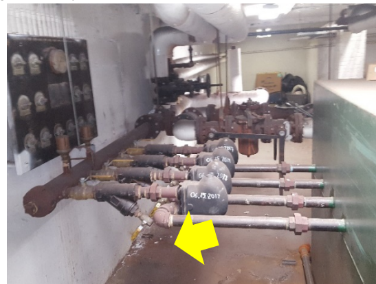
Un-insulated condensate pipes, steam traps and strainers (Ivy Hill Elementary School).
