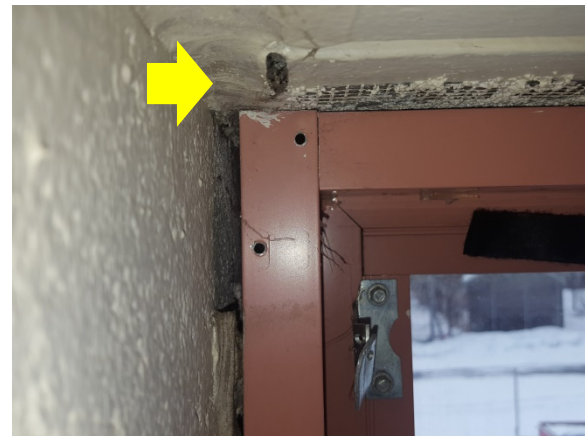
Buck Frame Air Sealing – above drop ceilings the window buck frame is often left untreated due to being out of sight. These areas of construction need be sealed to prevent air leakage just as the window trim and intersections are meant to be sealed below drop ceilings (Rafael Hernandez School).
