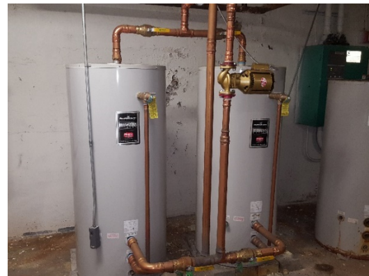
Un-insulated pipes in the domestic hot water system (Ivy Hill Elementary School).
