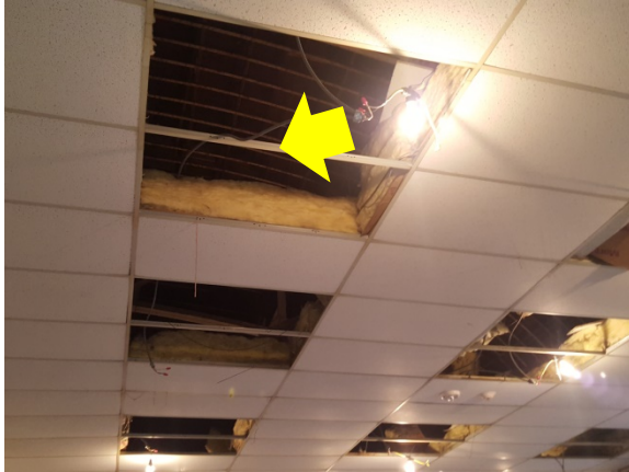
Attic Air Barrier Retrofit – failing ceilings above the drop ceiling expose the building to large amounts of air leakage. (Avon Academy).
