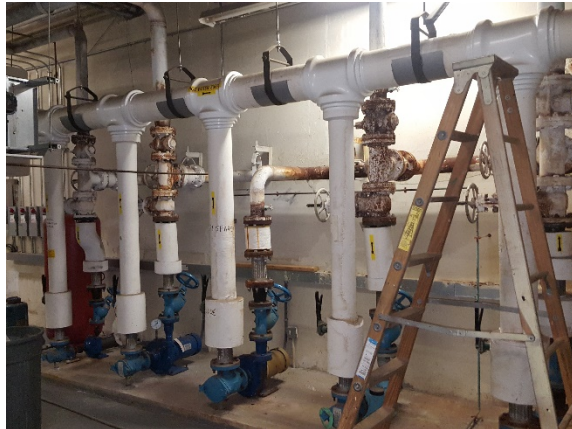
Suction diffusers, pumps and valves in the heating hot water system are not insulated (13th Avenue/ Dr. MLK Jr).
