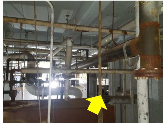
Un-insulated steam and condensate pipes (University High School).
