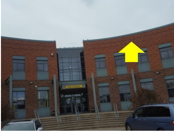
Roof-Wall Intersection Air Sealing – the exterior flashing and finishes at the roof-wall intersection are not constructed to stop air leakage (Belmont Runyon School).
