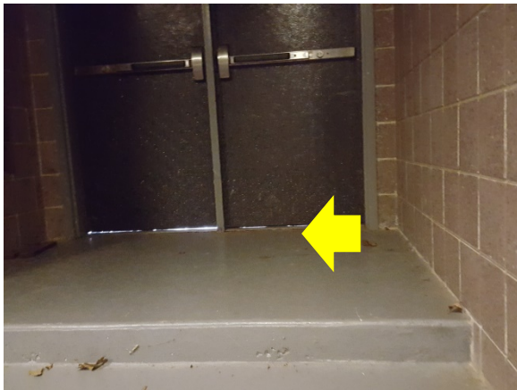
Door Weather Stripping – there are no door sweeps installed resulting in an obvious area of air leakage at the doors (Central High School).
