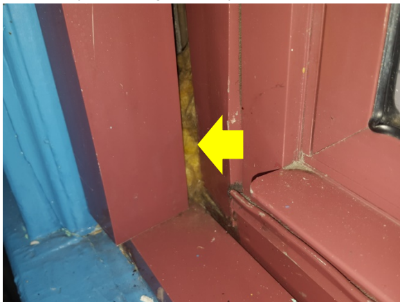
Caulking – unsealed snap trim with only air permeable fiberglass within the window cavity results in air leakage pathways around the window (South 17 th Street School)
