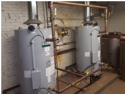
Un-insulated pipes in the domestic hot water system
