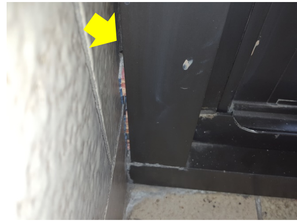
Caulking – unsealed snap trim reveal window framing components and dirt buildup at air leakage pathways around the window.
