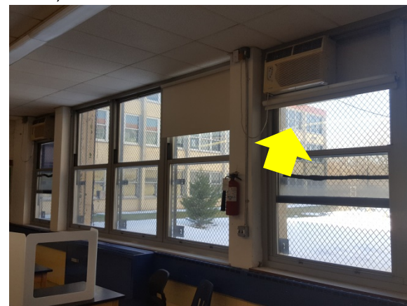
AC Unit Weatherization – the semi-permanently installed window AC creates a large gap old foam materials has deteriorated.
