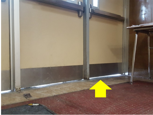
Door Weather Stripping – large gaps highlighted by daylights indicate air leakage pathways that need to be addressed in the building (Broadway/Luis Munoz Marin School).
