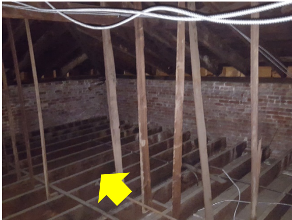
Attic Bypass Air Sealing & Insulation – there is no insulation at the attic flat. (Uplift/Newton School).
