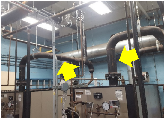
Un-insulated steam pipes (Branch Brook School/ ECC North).
