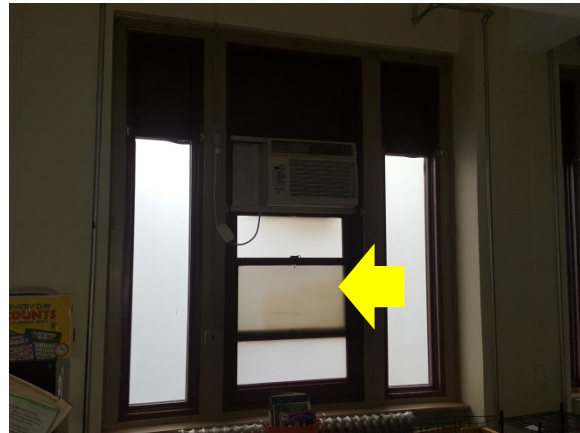
AC Unit Weatherization – the semi-permanently installed window AC creates a large gap between the window sashes where weather stripping at the meeting rail no longer makes contact (Lincoln Elementary School).
