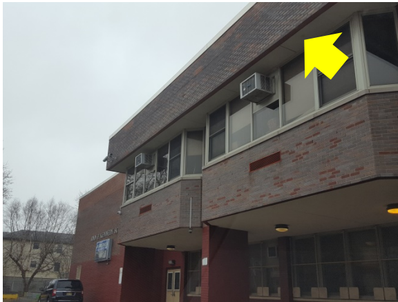
Overhang Air Sealing - the overhang extends beyond the conditioned space. Gaps in the exterior finishes of recessed lights and at perimeter of outdoor ceiling surface are direct pathways for infiltration/ exfiltration (John F. Kennedy School).
