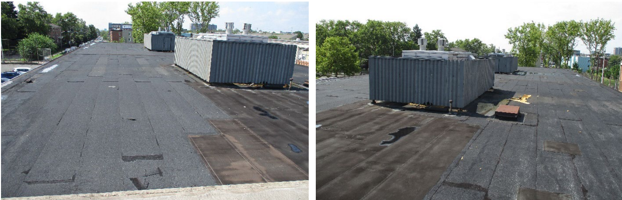
Seasons-4 Rooftop Multizone Units – ECC-Central
