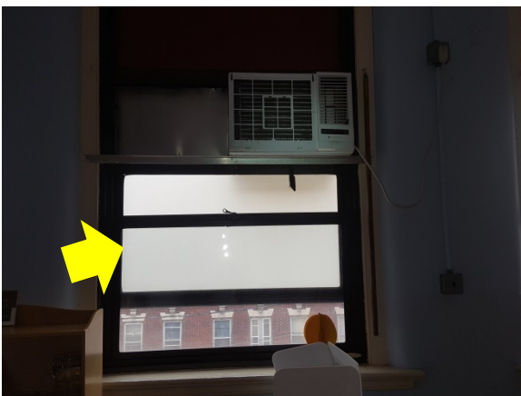
AC Unit Weatherization – the semi-permanently installed window AC creates a large gap (Abington Ave School)
