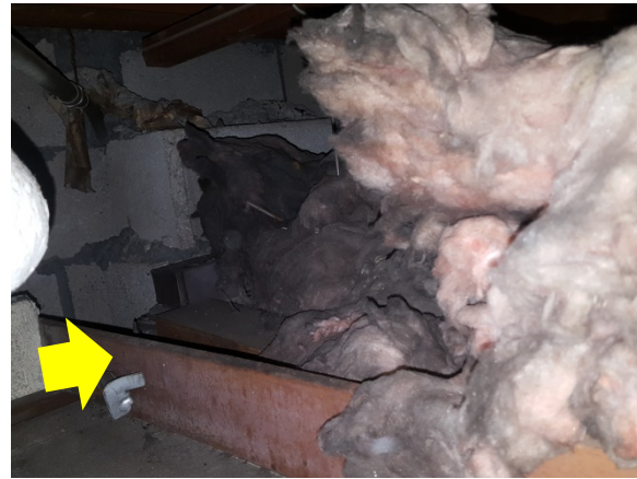
Overhang Air Sealing – the plane of the exterior wall does not extend beyond the drop ceiling. Dirt buildup in fiberglass indicates air leakage as fiberglass “filters” debris as air moves through the building envelope (Bard Early College School).
