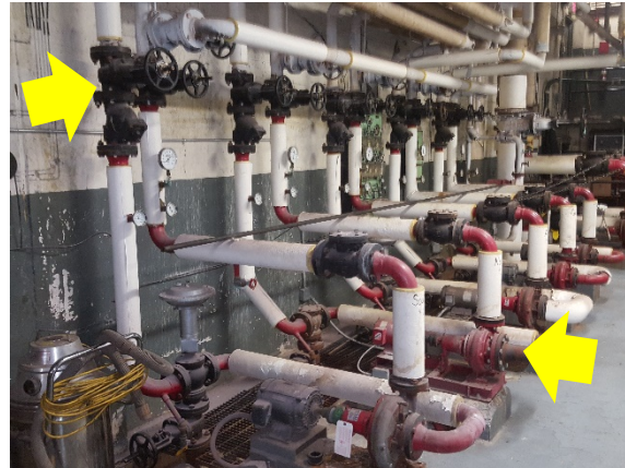
Pumps and valves in the heating hot water system are not insulated (McKinley School).
