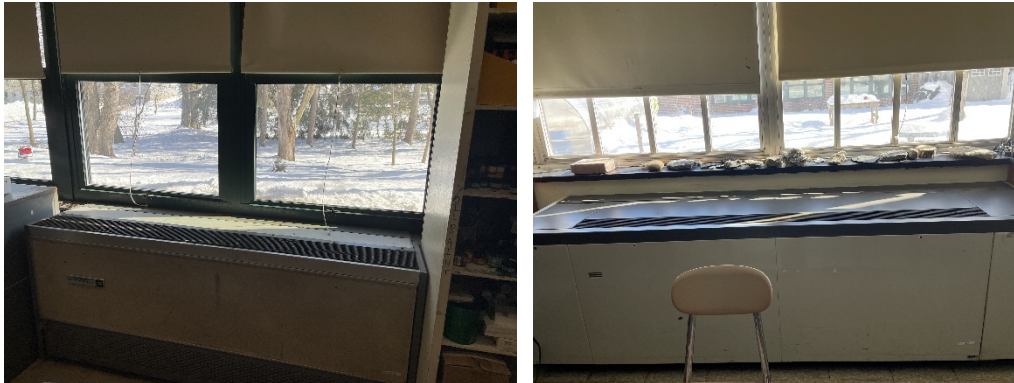
Existing unit ventilators at Passaic Valley Regional HS
