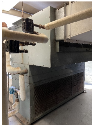
Existing air handling unit at Passaic Valley Regional HS
