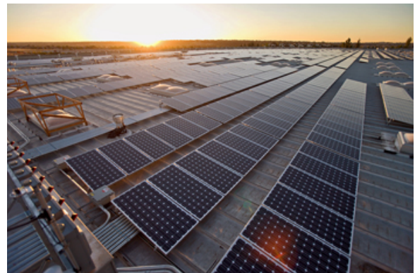
Photovoltaic (PV) solar array
