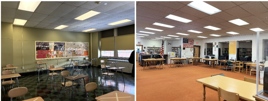
Existing interior lighting at Passaic Valley Regional High School
