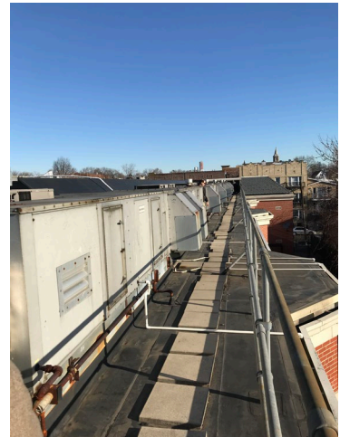
Figure 6. Bethune HVAC Equipment
