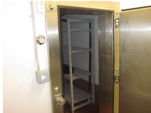
Walk In Refrigerator – South Kitchen
