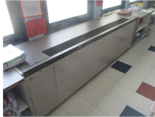
Watching Hills – South Building Univents
