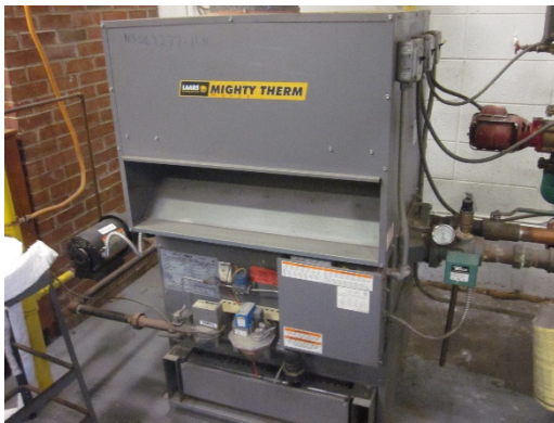
Kitchen Water Heater
