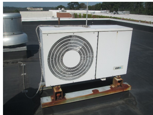
Split Units – West Wing
