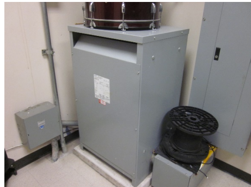
Transformer – Watchung Hills RHS
