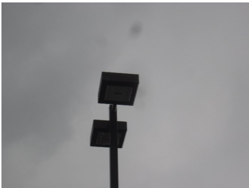
Existing Outside Lighting
