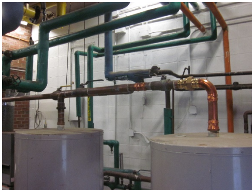
Uninsulated Piping – South Kitchen Water Heater
