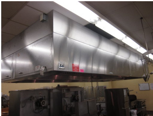
Kitchen Hood – North Kitchen
