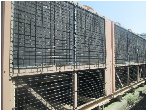
Chiller 1 – South Building
