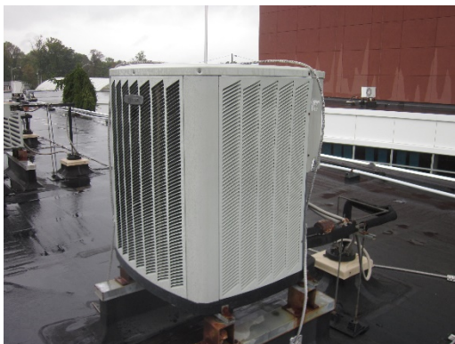
Split Units – West Wing
