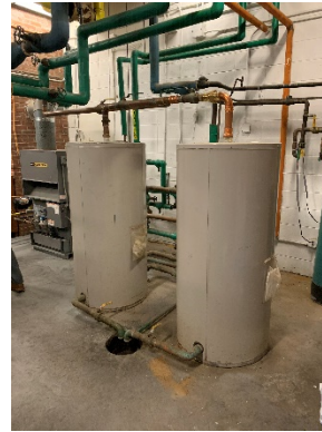
Uninsulated Piping – South Kitchen Water Heater
