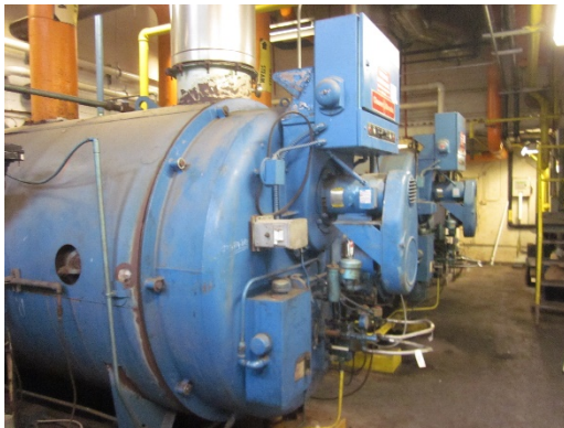
North Boiler Room
