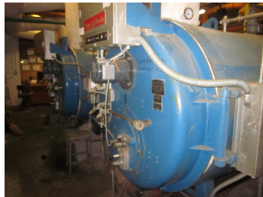
South Boiler Room
