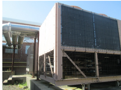
Chiller 2 – South Building
