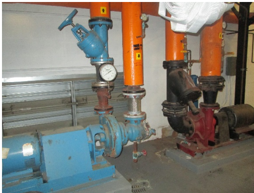
North Wing HHW Pumps
