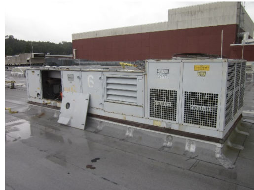
Nesbitt Roof Top Unit
