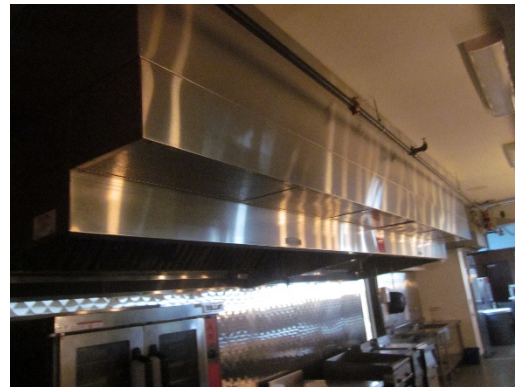
Kitchen Hood – South Kitchen
