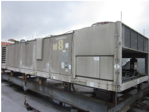
McQuay Roof Top Unit
