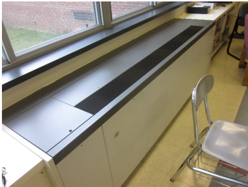
Watching Hills – South Building Univents
