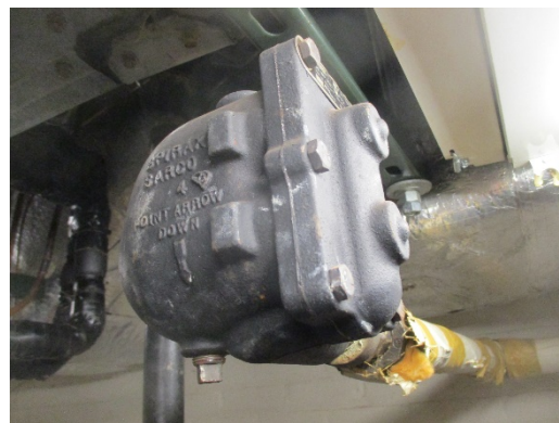
Watchung Hills RHS Steam Trap
