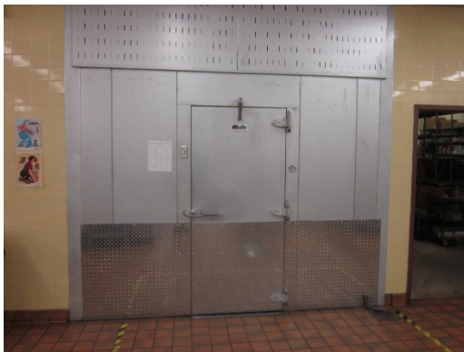
Walk In Freezer/Refrigerator – North Kitchen
