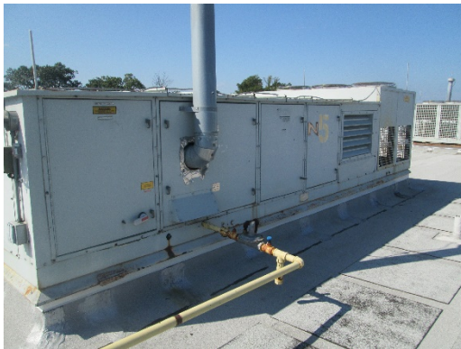
Watchung Hills RHS -RTU
