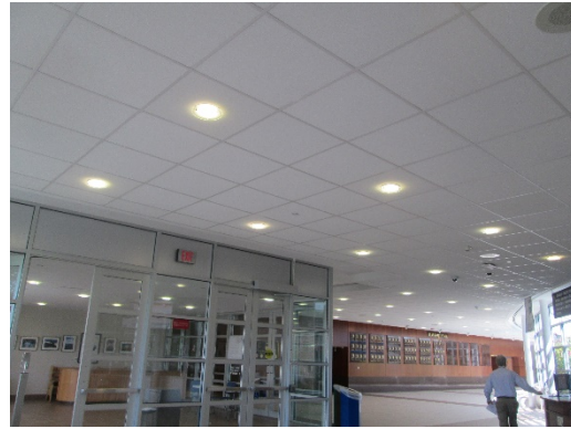
Existing Lighting Main Entrance
