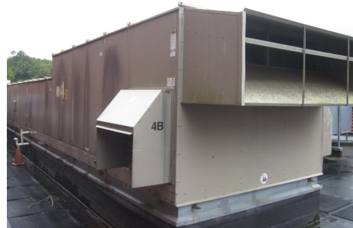
Watchung Hills RHS -RTU
