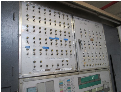
Watchung Hills RHS Controls
