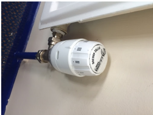
Radiator TRV Valve
