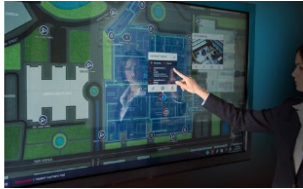
HVAC Equipment Control
