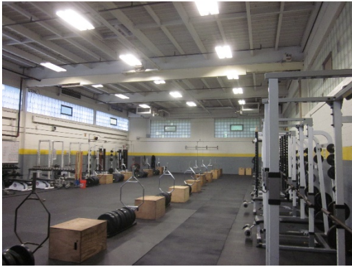
Existing Lighting at Weight Room 3-4
