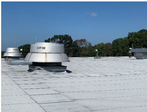
Watchung RHS – Exhaust Fans
