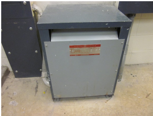
Transformer – Watchung Hills RHS
