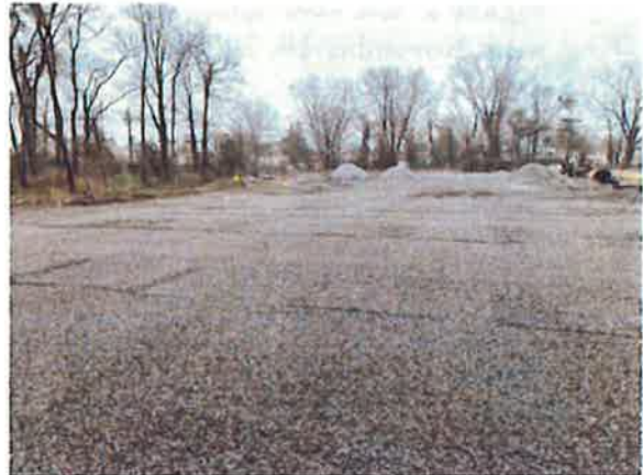
Figure 8. Gravel laid out and raked for solar racking system to be placed March 24, 2022
