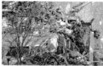
Cleanup begins in January after a massive fire consumed the Avalon at Edgewater. Proposed legislation would ban construction such as that used at the luxury complex in certain communities. (JAVANIA MARQUEL/COM ADVANCE MEDIA/GETTY IMAGES FOR THE STAR-LEDGER)
